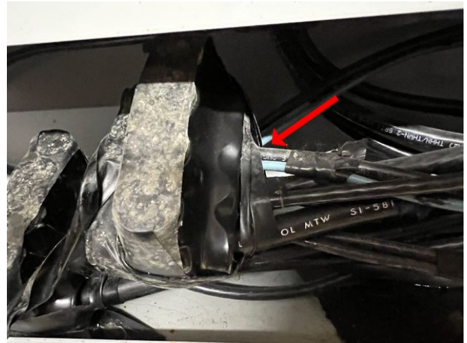
Double lugged terminals at gutter cabinet
