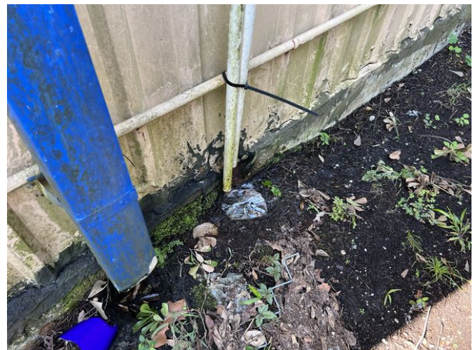
A/C drain lines deposit right side building
