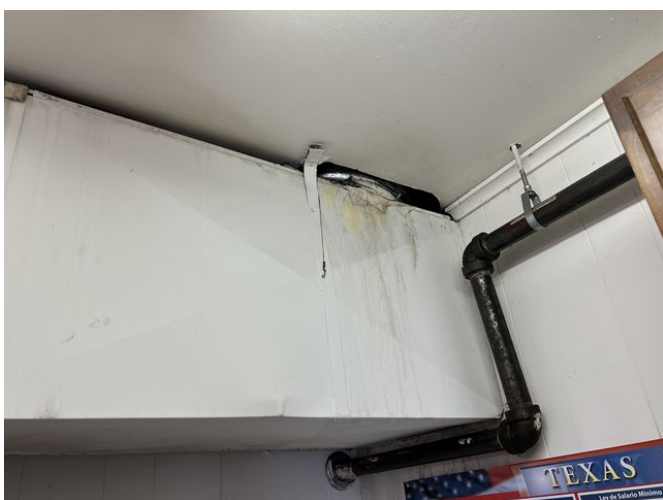
Duct sweating at receiving room
