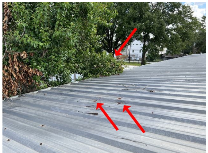
Rust at roof covering, vegetation contact right slope
