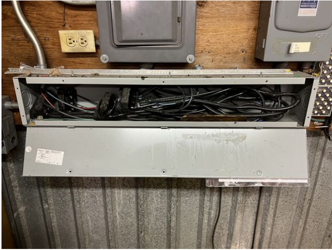
Grounding and bonding not originated at service gutter
