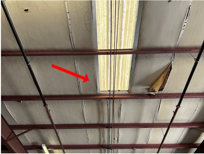
Skylight leaking left roof slope
