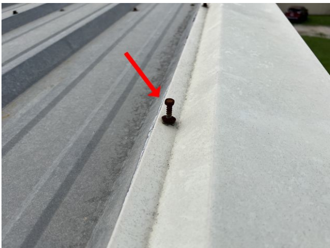
Loose fasteners at roof covering
