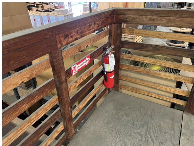
Fire extinguisher at the attic stairway landing
