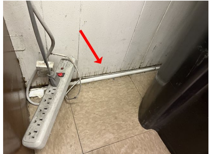
Moisture stains receiving room front wall
