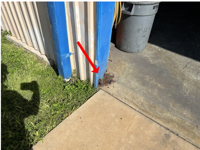
Deteriorated jamb warehouse garage door
