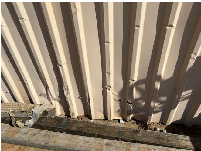
Damaged siding from equipment contact
