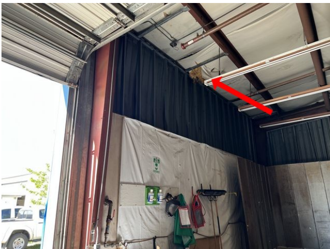
Leak at left rear corner warehouse
