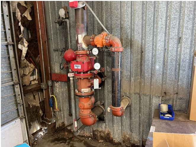
Fire sprinkler controls at warehouse
