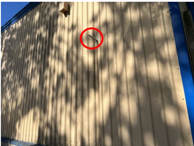
Auxiliary drain line not a conspicuous location
