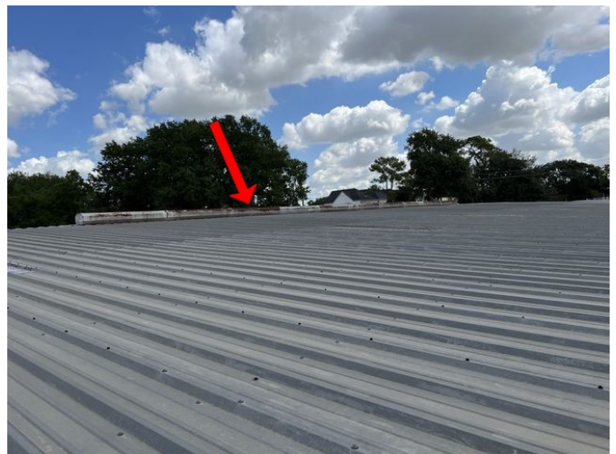
Rust along the ridge cap
