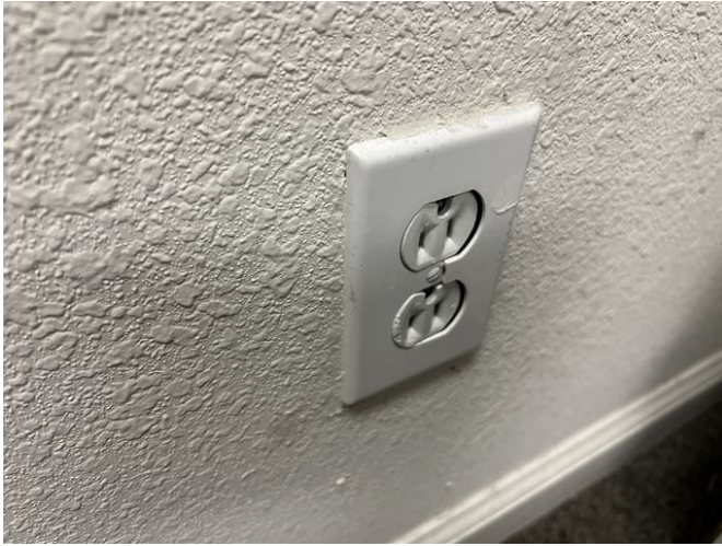
Several of the coverplates are cracked in the offices
