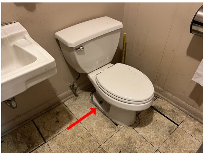
Commode loose at floor storage room bathroom
