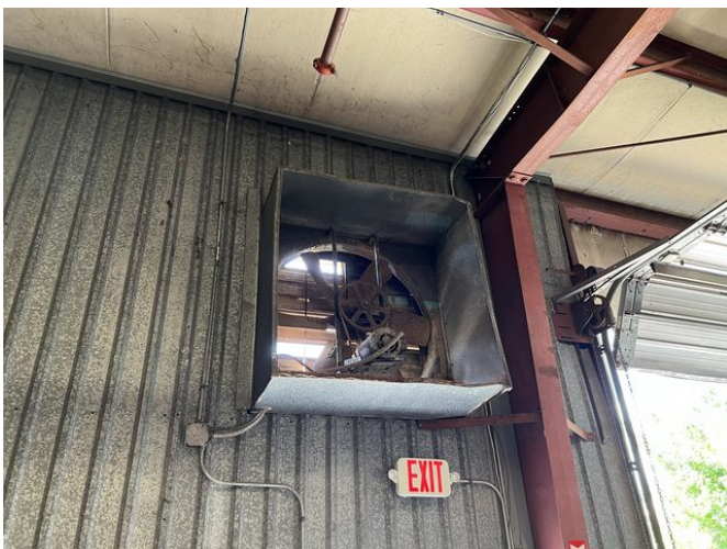
Warehouse left wall ventilation fan not working
