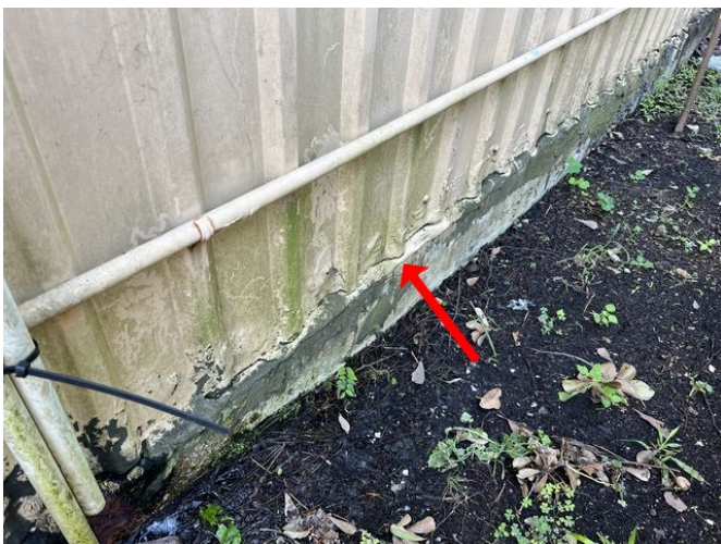
Siding not flashed at the slab, tar applied in places
