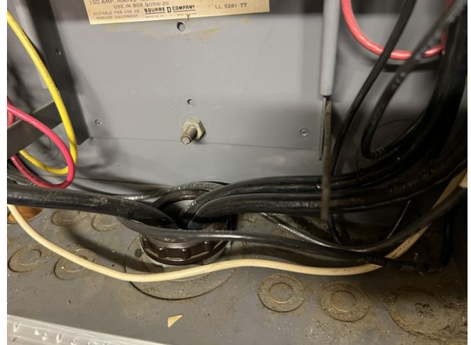
No ground from the gutter cabinet point of service
