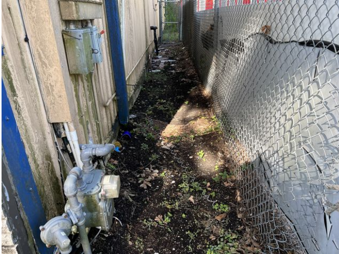
Improper grading right building
