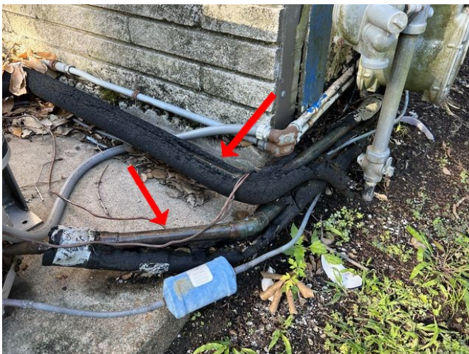
Deteriorated suction line insulation at exterior
