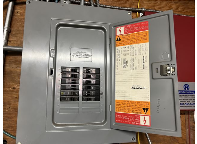
Labels missing at the dead front cover
