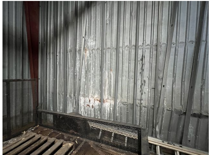
Metal stud damage right warehouse wall, siding rusted
