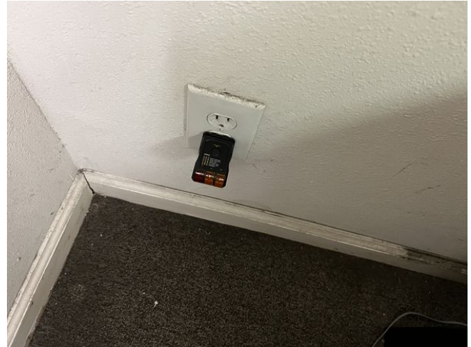
No power reception left wall receptacle
