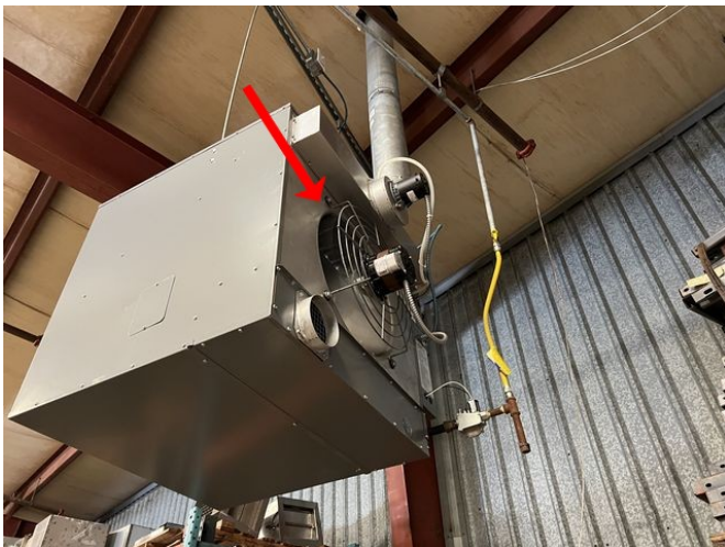
Fan vibration right warehouse heater when operated
