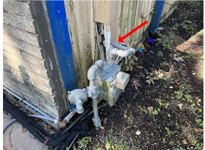
Gas pipe not bonded right side building
