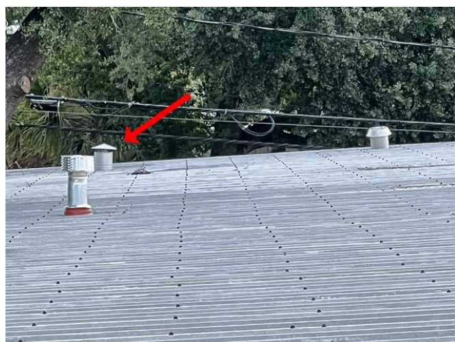
both furnace are not properly vented to the exterior
