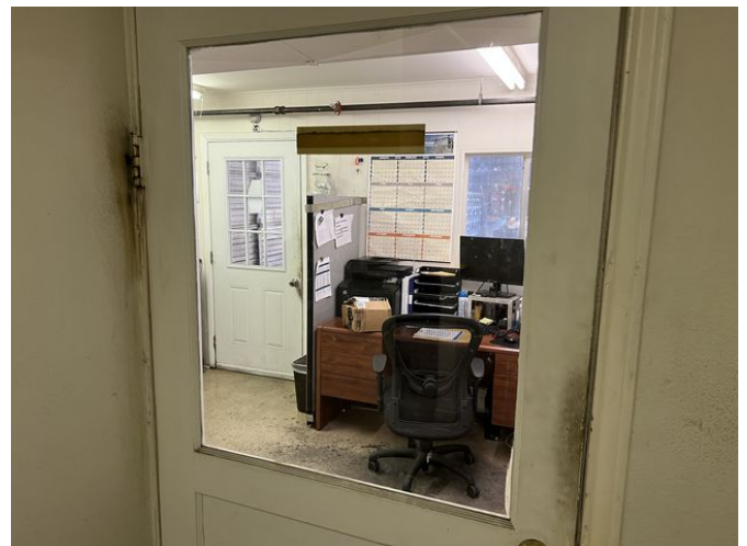
Glass not tempered at hallway door at receiving room
