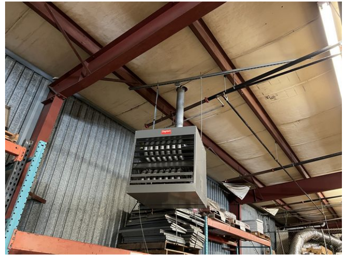
Right warehouse heater
