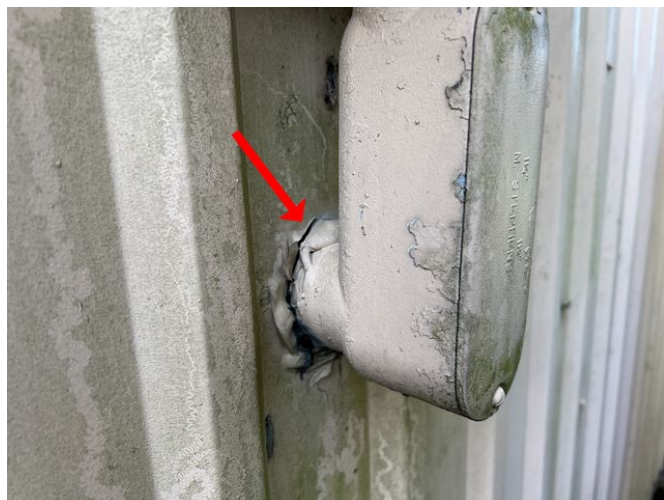
Penetrations not properly sealed
