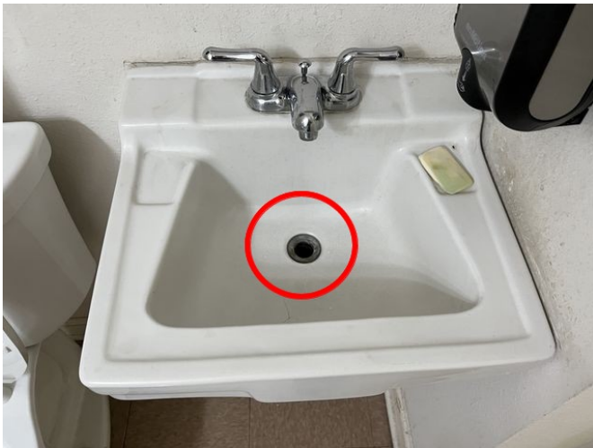
Sink stopper missing men's bathroom
