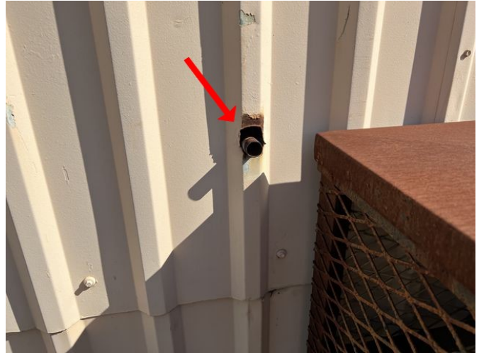
Penetrations not sealed several locations
