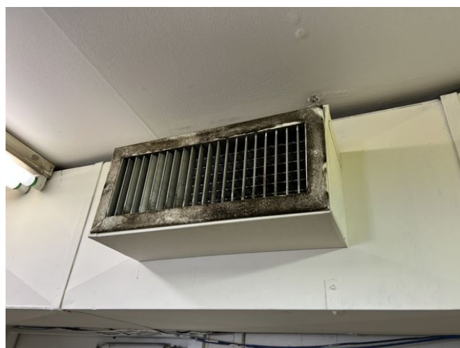
Organic stains observed at receiving room register
