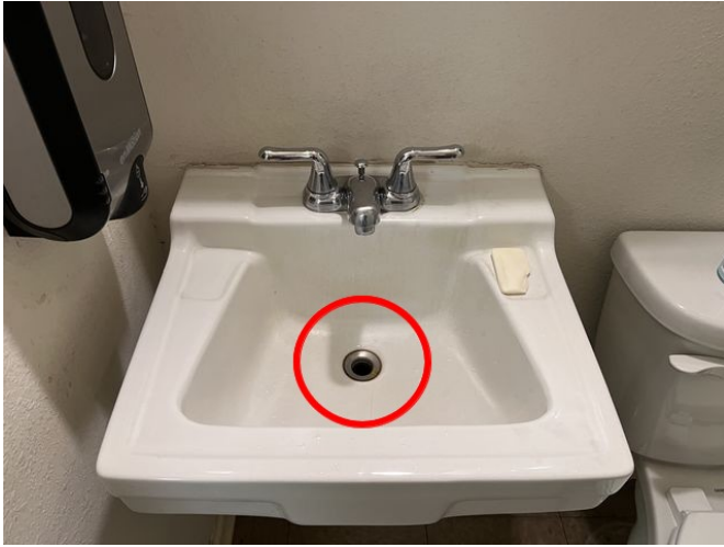
Sink stopper missing women's bathroom
