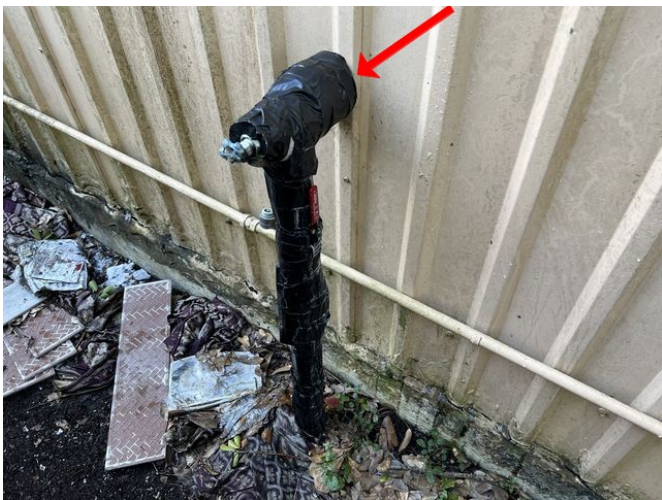
Galvanized water pipe not bonded right side building
