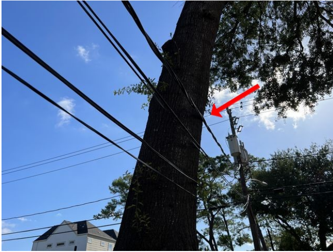
Power lines in contact with front tree
