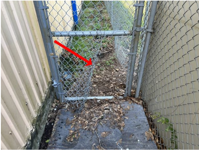
Gate damaged right side building
