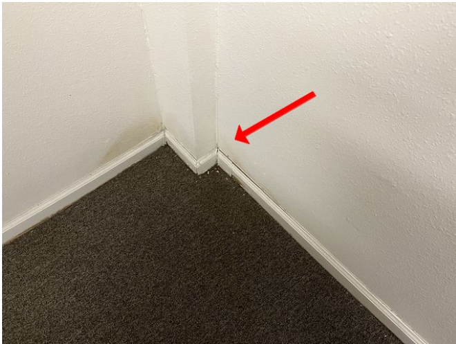
Moisture stains right front office base wall
