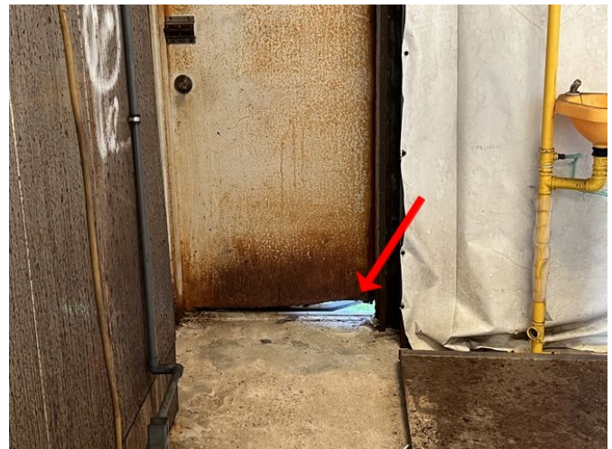
Rear warehouse door deteriorated
