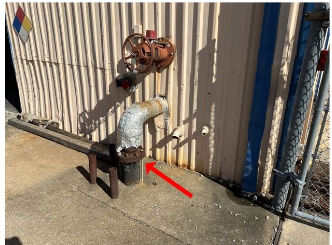
Insulation missing at sprinkler main waterline
