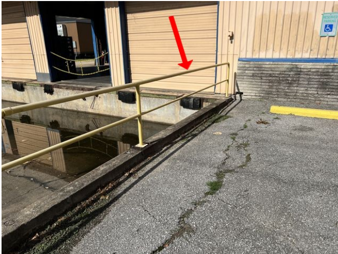
Delivery well guard rail has opening wider than 4"
