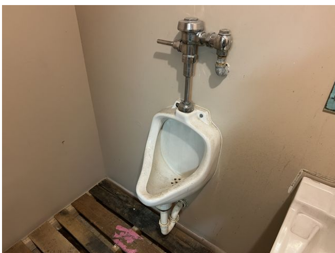
Urinal not working at storage room bathroom
