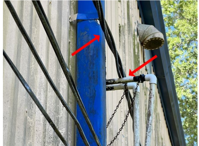
Power lines on the A/C drain lines, clearance gutter
