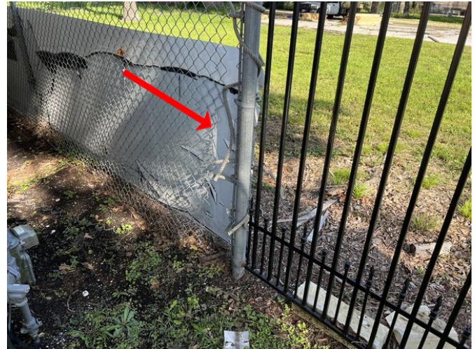
Right property line fencing damaged
