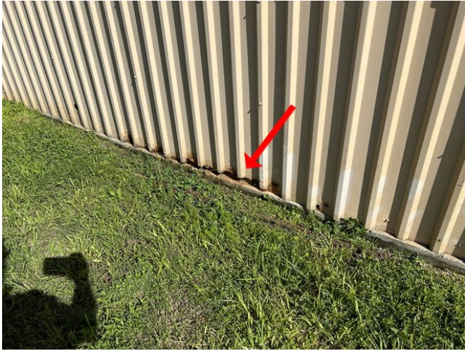
Rust at the base of the walls at several locations
