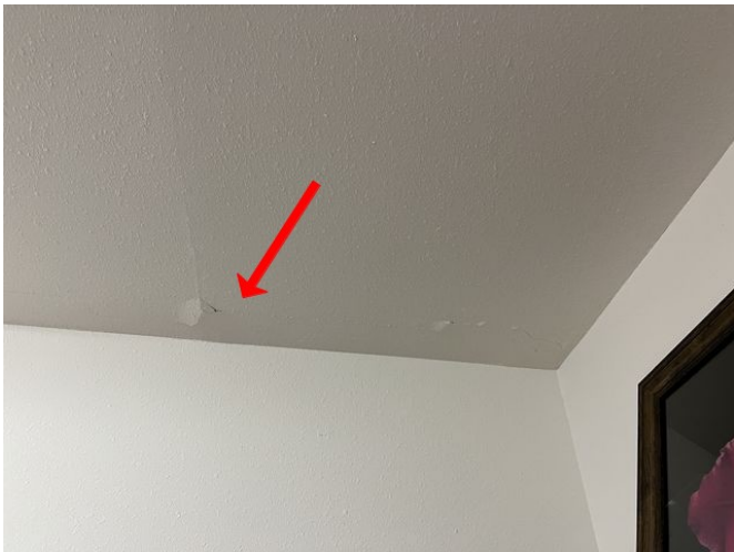
Drywall cracked rear office ceiling
