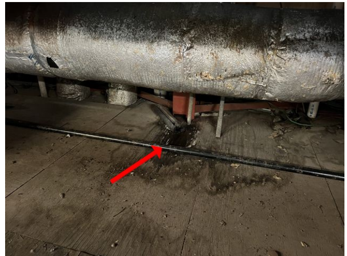
Ductwork sweating and dripping at attic
