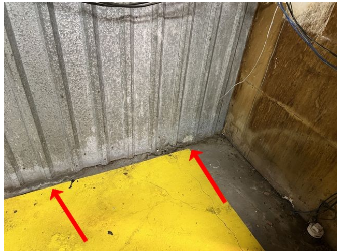
Moisture stains storage room floor at right wall
