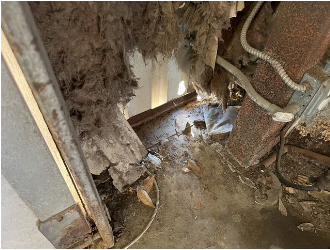
Hole siding front building, insulation missing
