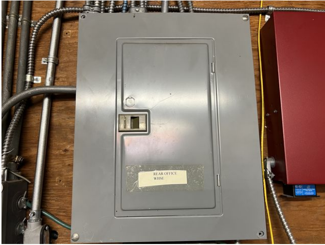
Right panelboard, Square D
