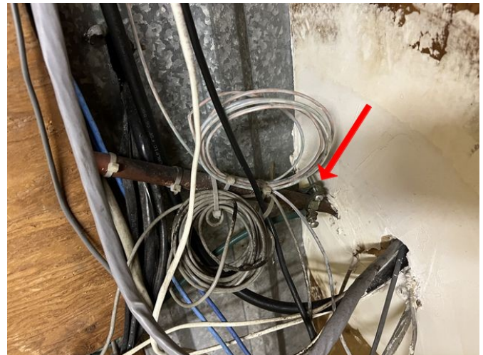
Metal building bonding clamp at storage roof
