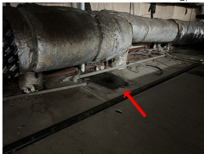
Ductwork sweating and dripping at attic
