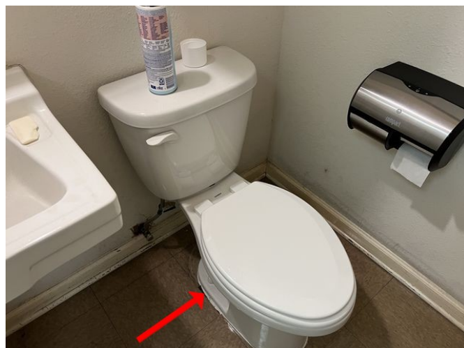
Commode loose at floor women's bathroom
