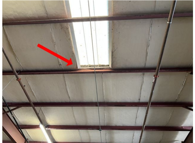
Skylight leaking left roof slope
