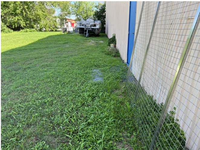
Inadequate slope rear building
