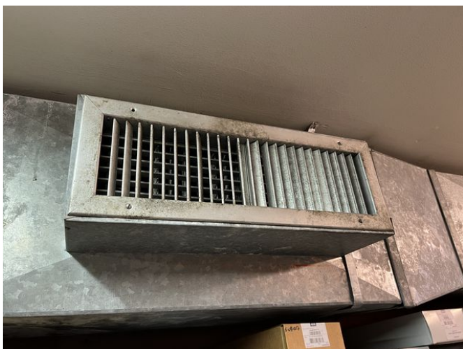
Organic stains observed at storage room registers
