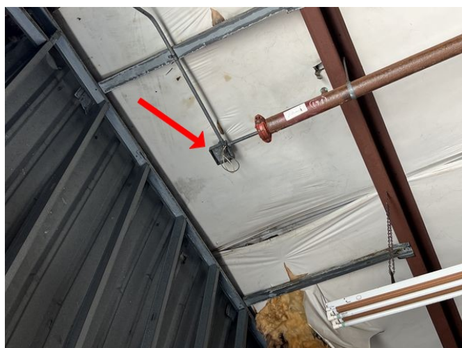
Junction box coverplate missing at warehouse ceiling
