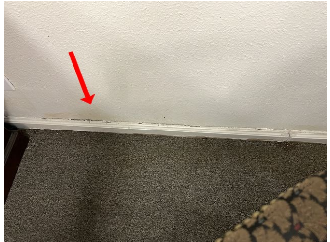
Moisture stains right front office base wall
