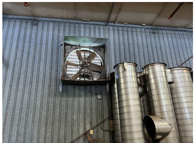
Warehouse right wall ventilation fan not working
