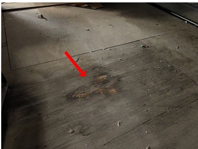
Ductwork sweating and dripping at attic
