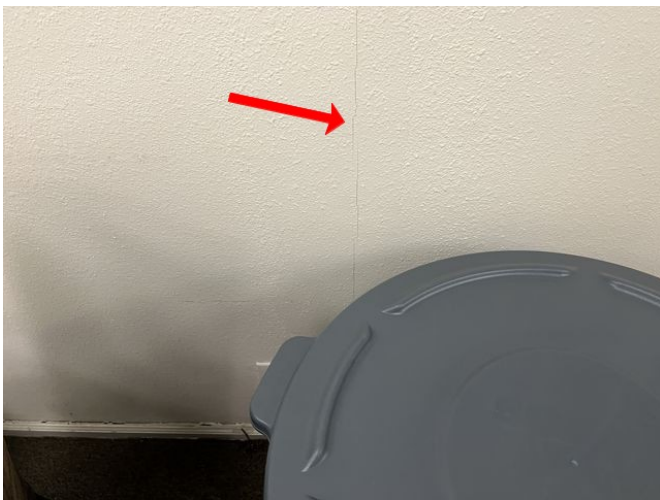
Drywall crack right front office right wall
