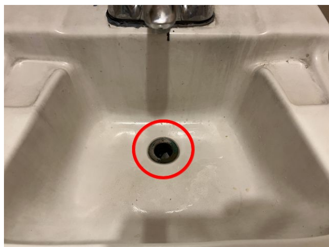
Sink stopper missing storage room bathroom
