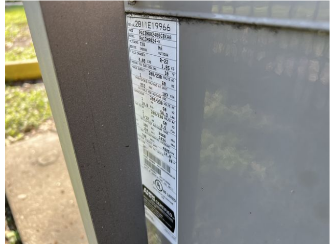
Storage area condensing unit labeling, 2 tons
