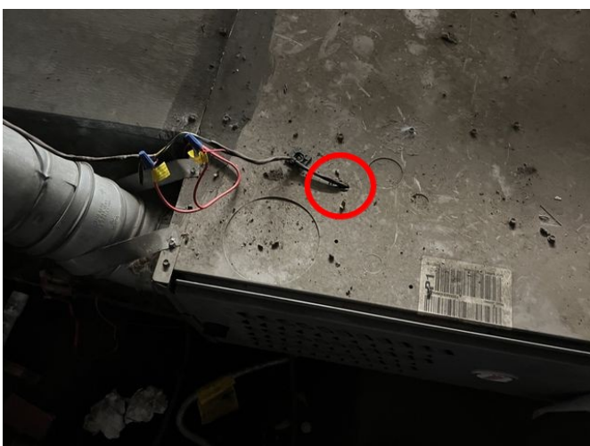
Thermostat wires not sleeved at storage area furnace
