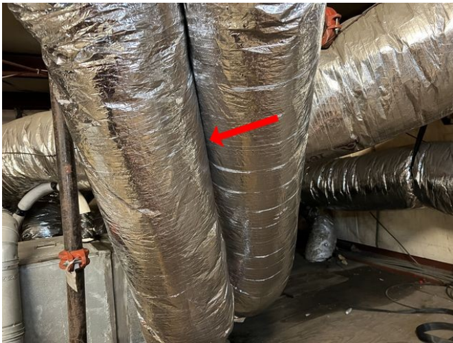
Separate ductwork where touching at attic
