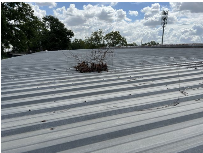
Debris right roof slope
