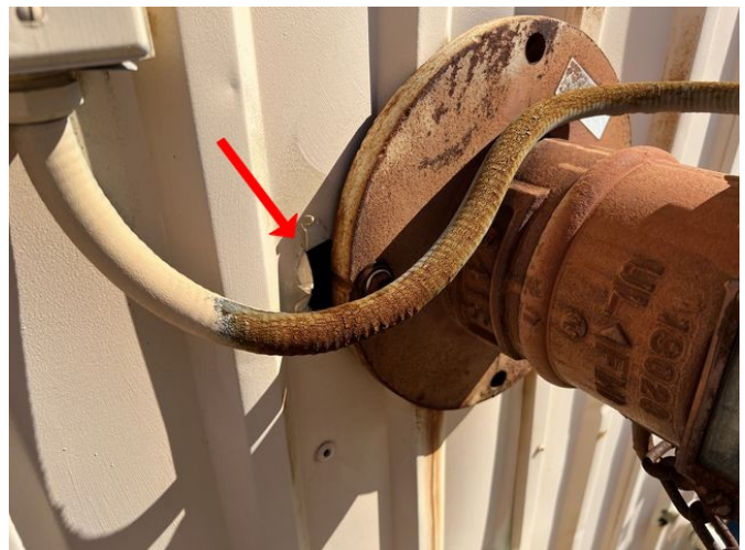
Penetrations not sealed at siding
