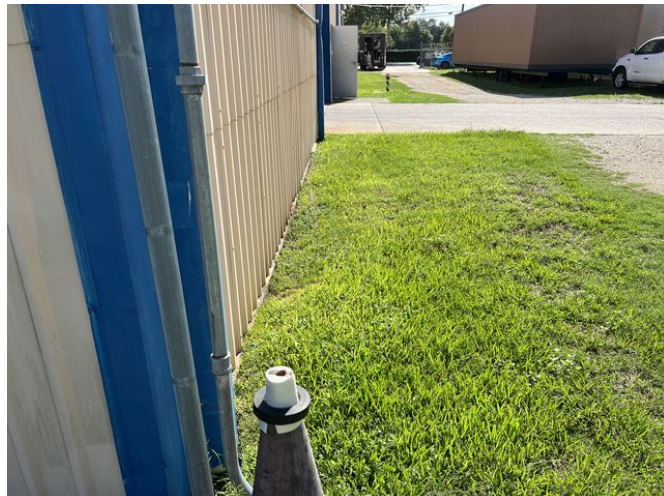
Inadequate slope left rear building
