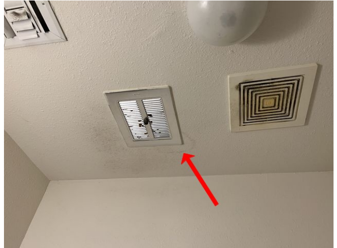
Moisture stain women's bathroom ceiling
