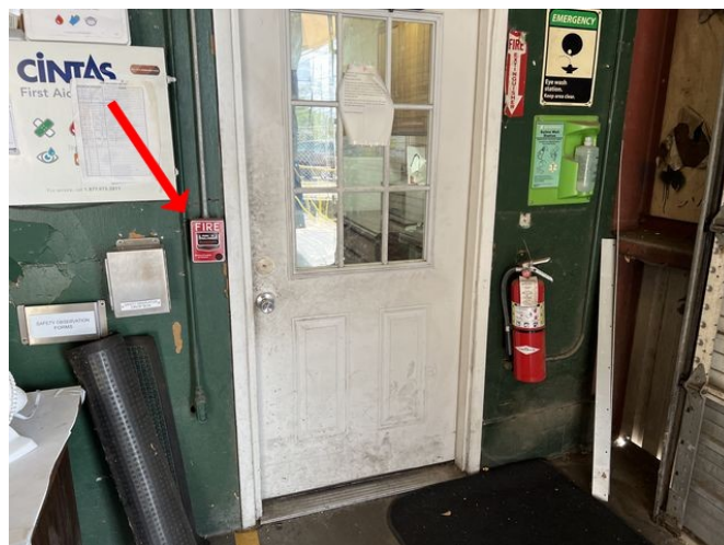
Manual fire alarm lever at receiving door
