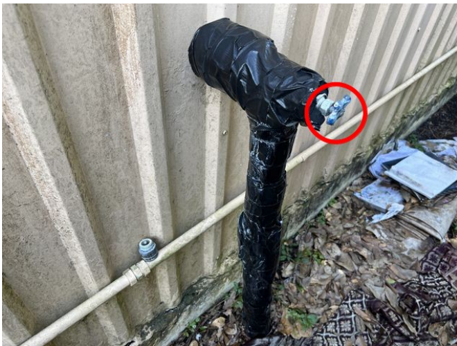
Broken wheel handle right hose bib
