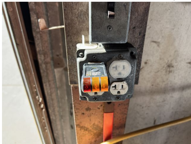
No GFCI receptacles installed in the warehouse
