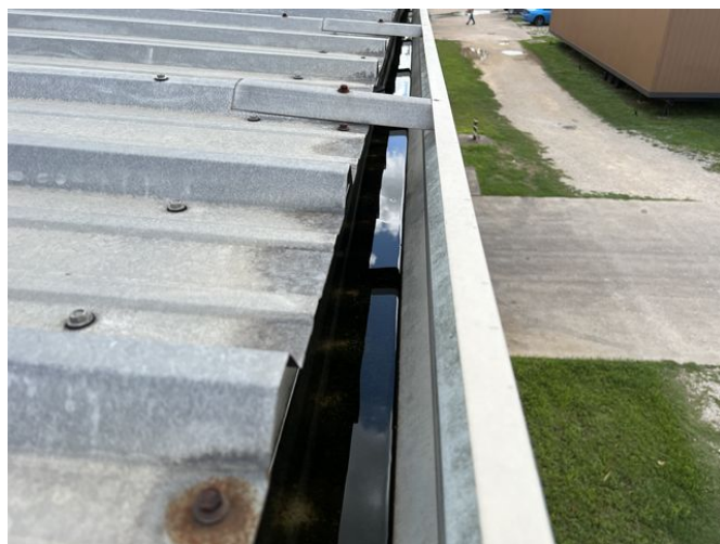
Standing water gutters
