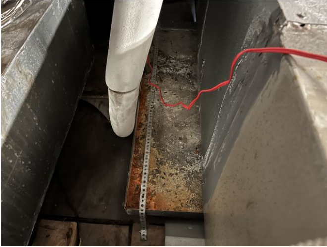
Office A/C drain pan rusted, monitor
