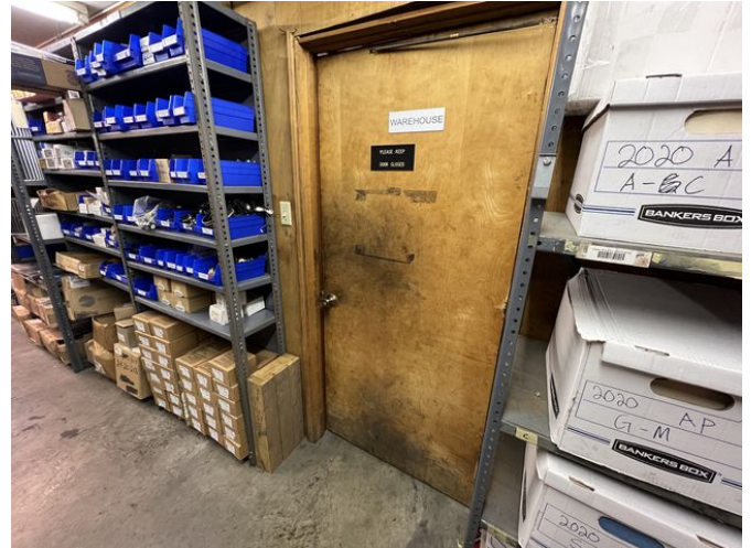
Storage room rear door not weather stripped
