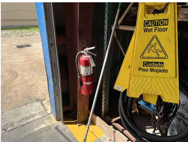
Fire extinguishers located at the exterior doors
