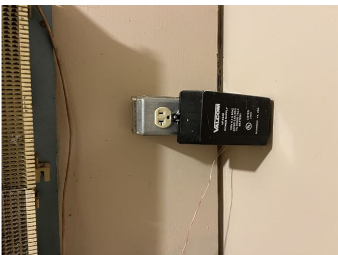
No GFCI receptacles installed at the bathrooms
