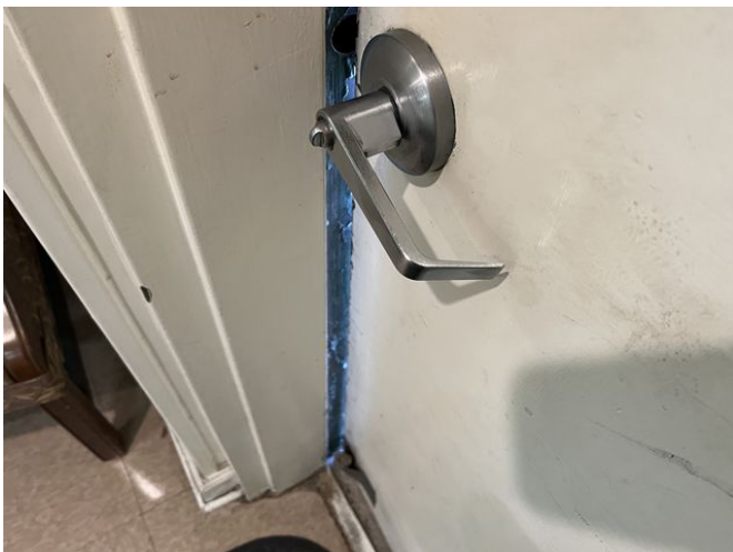
Front entry door not weather stripped
