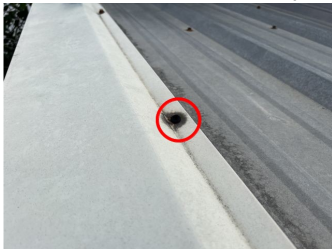
Missing fasteners at roof covering
