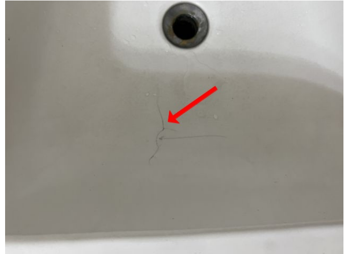
Sink bowl cracked men's bathroom
