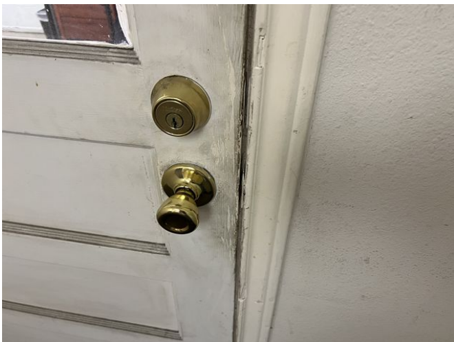
Office hallway door at receiving room not latching
