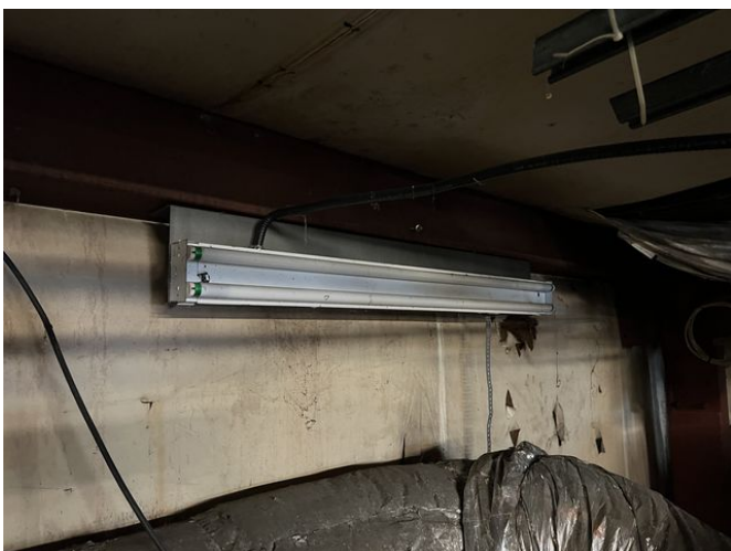
Attic light at the right wall not working
