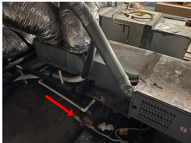
Gas shut off valve too far from the office furnace
