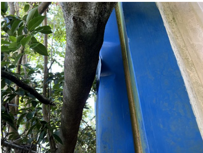
Tree contact siding right rear building
