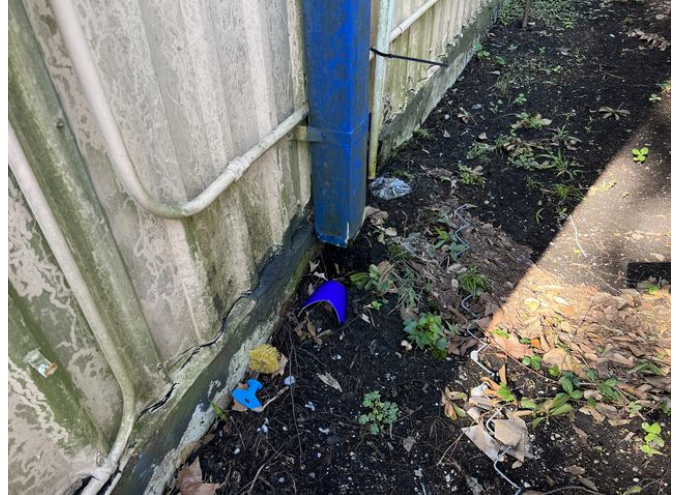
Downspouts missing diverters and splashblocks, erosion
