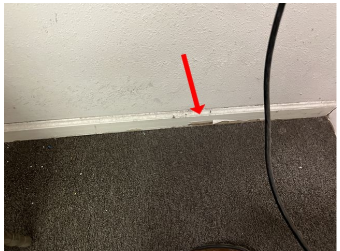
Moisture stains receptionist room front wall
