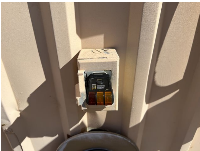
No GFCI receptacles at the exterior
