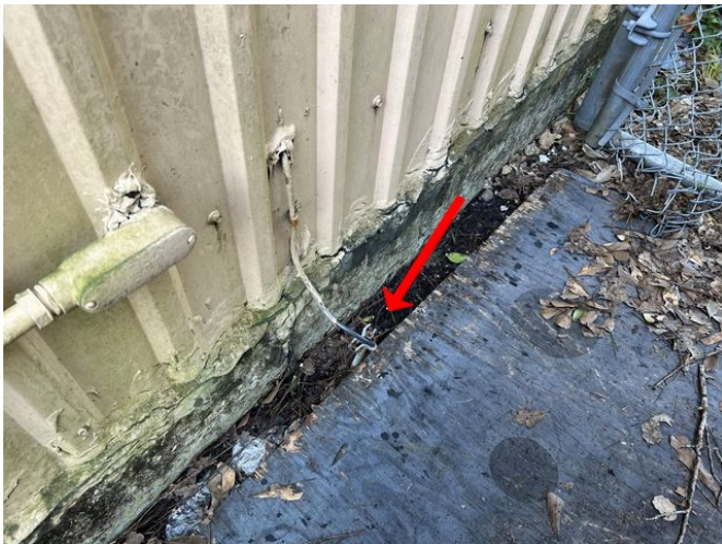
Ground rod at right side building not driven below grade
