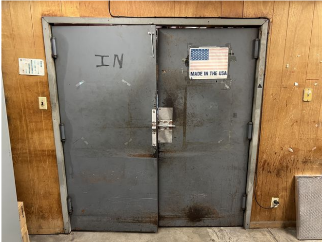
Storage room rear double doors not weather stripped
