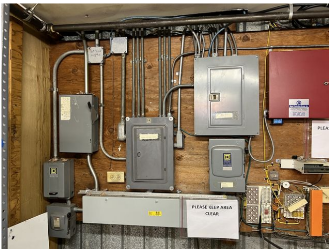
Building electrical service at the storage roof
