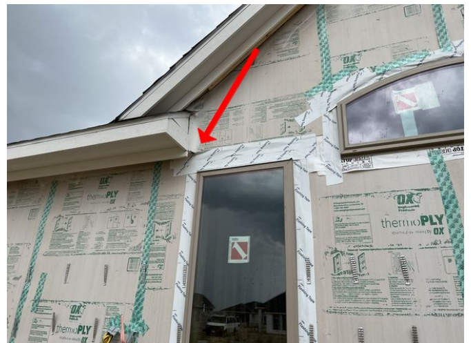
Loose flashing tape above dining room window
