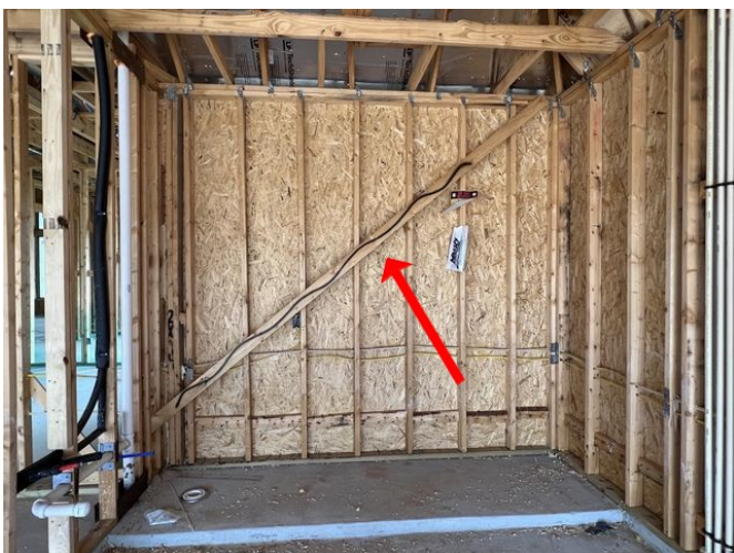
Temporary brace not removed rear garage wall
