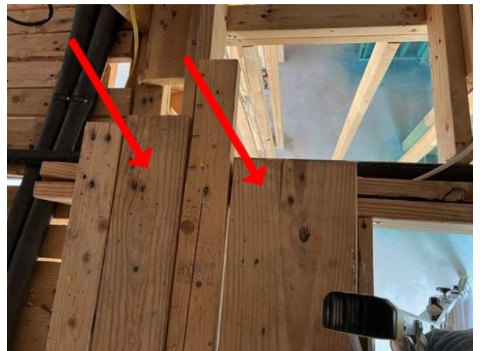
Nails missing decking top ladder access opening
