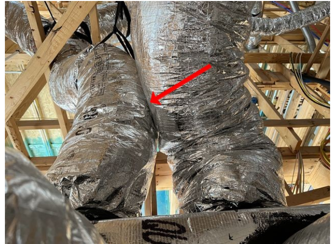
Separate ductwork where touching at attic
