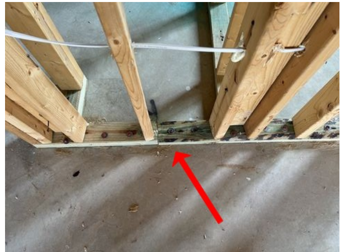
Joint not blocked garage rear wall toe plate
