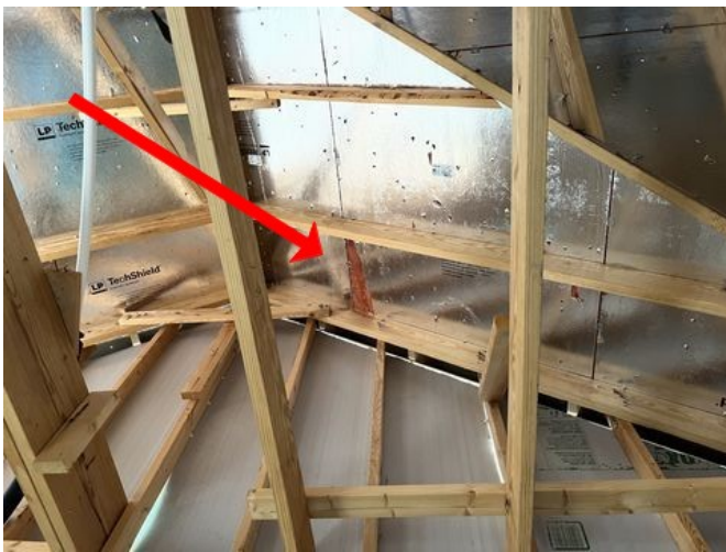
Damaged radiant barrier above left front bedroom
