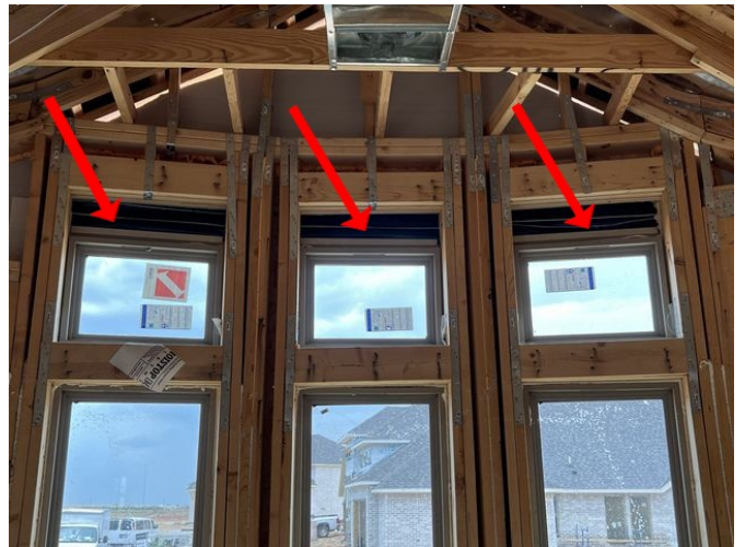
Master bedroom clearstory windows not poly sealed
