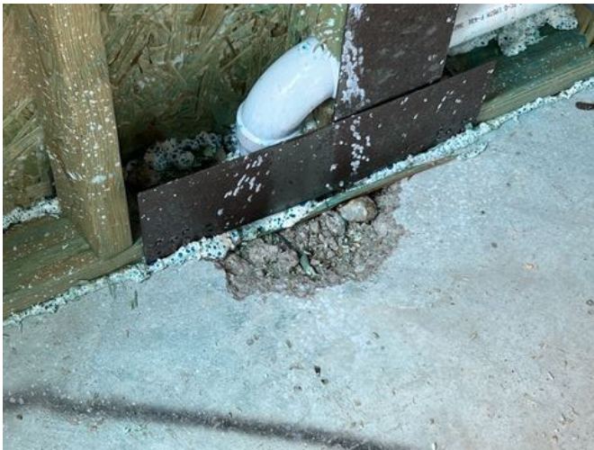
Slab not patched at master bedroom right wall
