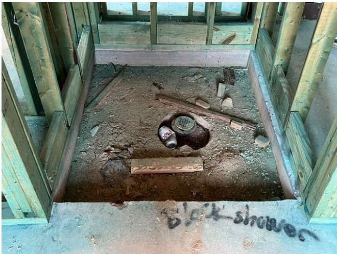
Shower liner missing at master bathroom
