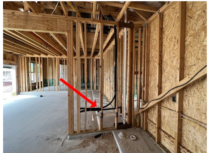
Double stud not continuous at garage sink drain
