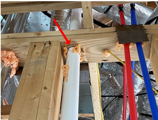
Seal plumbing penetration right front bathroom
