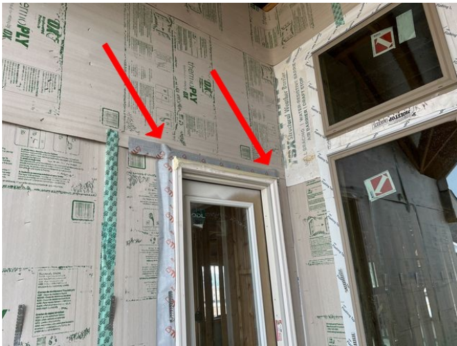
Loose flashing tape above rear patio door
