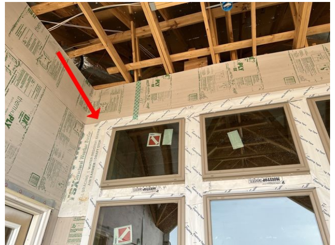
Loose flashing tape above family room window
