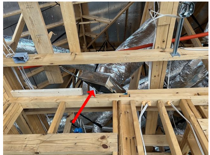
Return air box not secured right front bedroom
