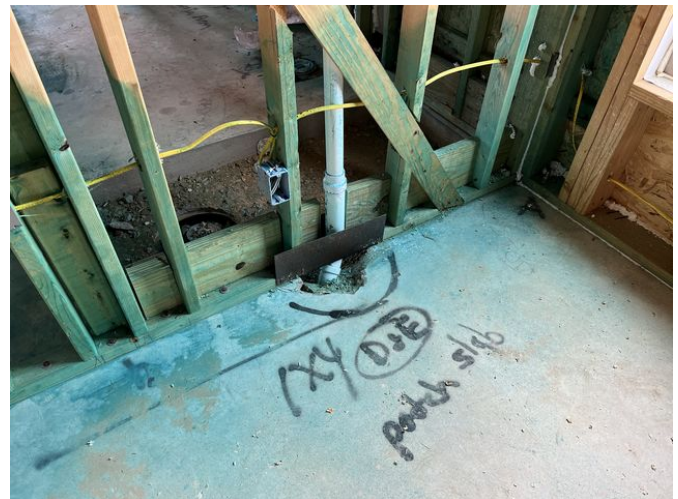
Slab not patched at dining room floor
