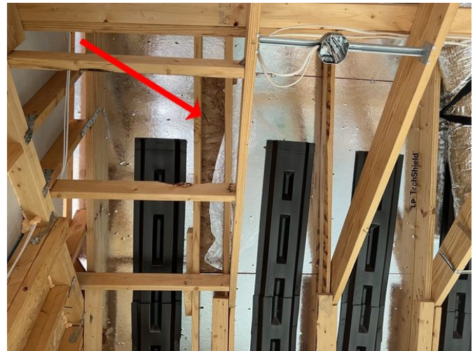
Damaged radiant barrier above right rear bedroom
