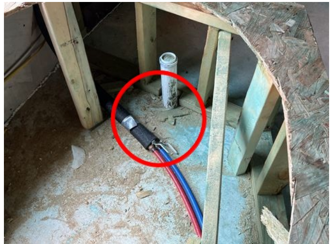
No drain well present at master tub
