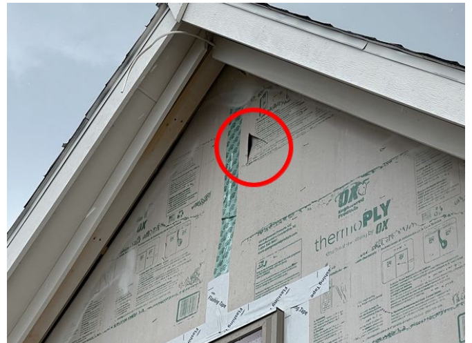
Hole T-ply at garage gable
