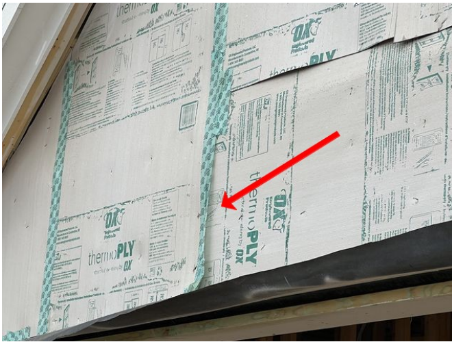
Loose flashing tape above the garage double door
