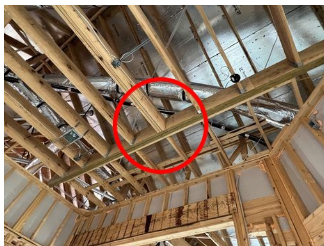
Joist hanger missing above kitchen at beam intersection
