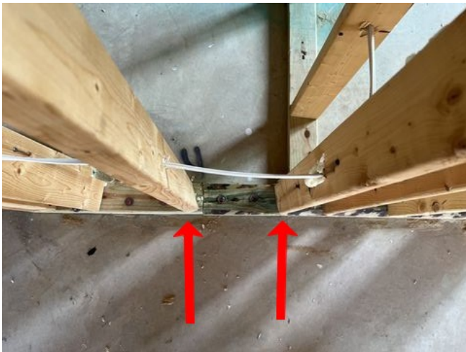
Studs twisted base rear garage wall
