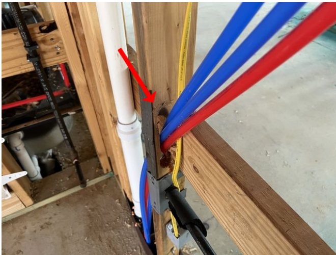
Stud boring excessive utility room rear wall
