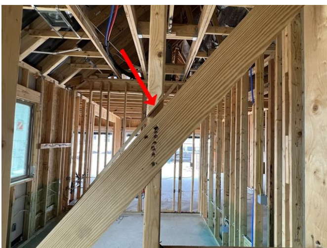
Studs over notched at LIB at front office wall
