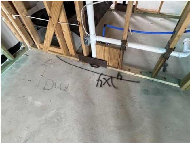
Slab not patched at right rear bedroom floor
