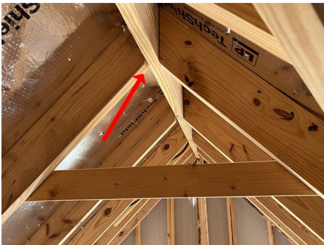
Ridge brace undersized at garage gable
