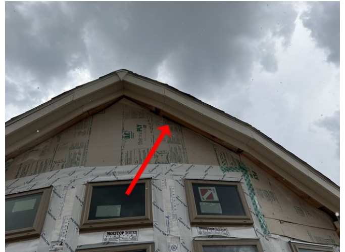
Gap in the T-ply rear master gable
