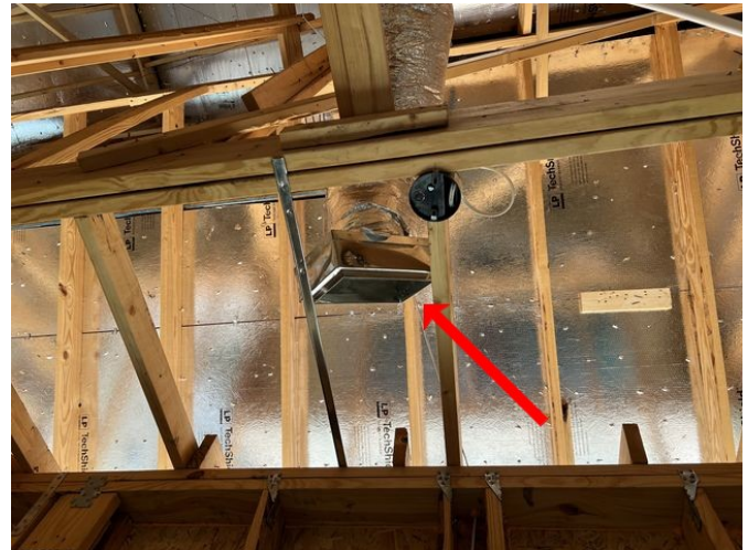
Air supply register not secured left front bedroom
