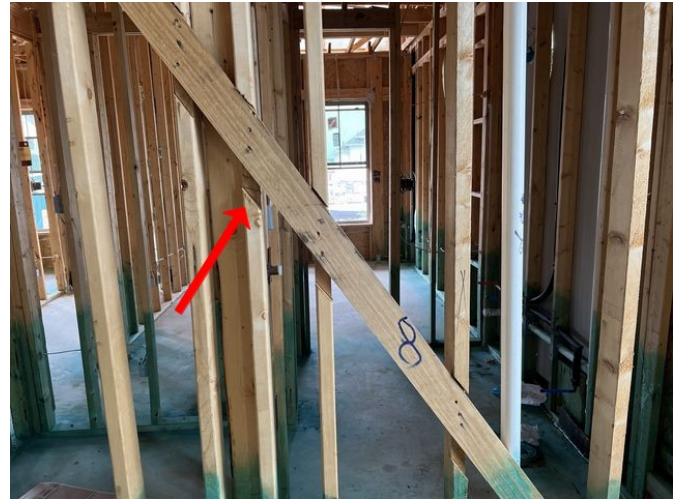
Studs over notched at LIB left front bedroom
