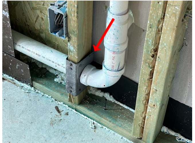
Nails missing at stud boot master bedroom right wall
