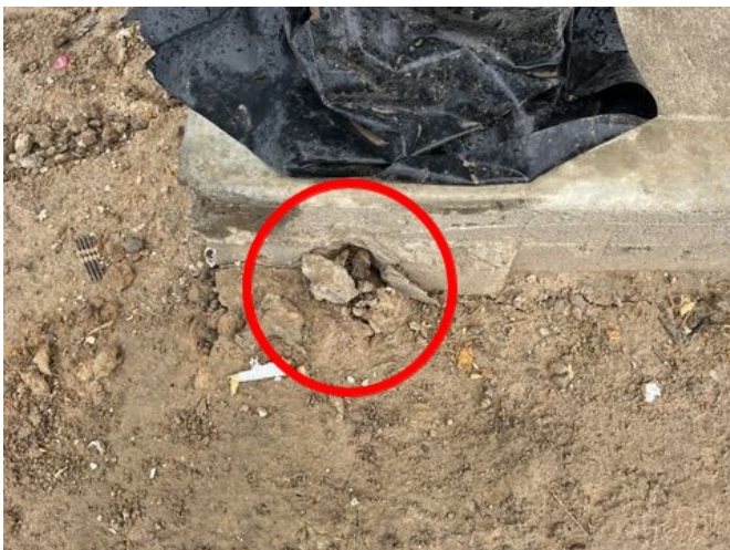
Post tension cable blow out left front dwelling
