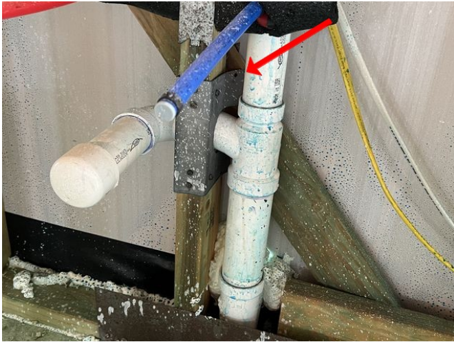
Nails missing at stud boot left master bathroom sink
