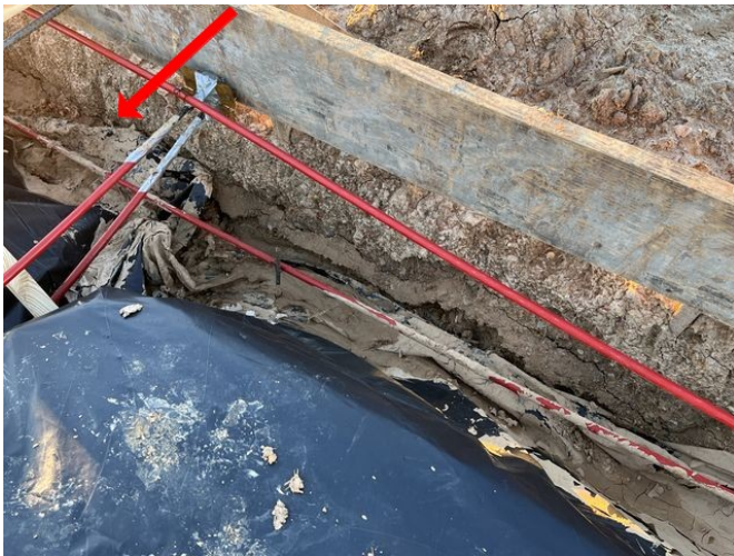
Cave-in/erosion at left perimeter beam
