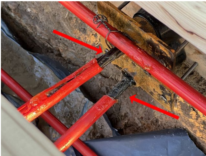
Cables not properly covered at the perimeter ports
