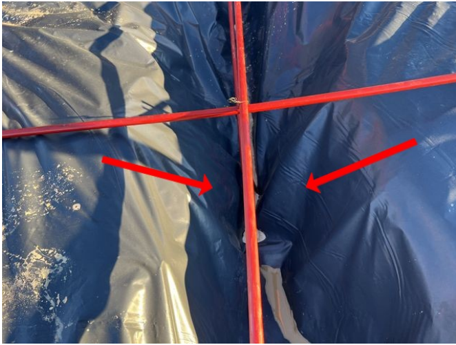
Poly not covering the bottom of the garage interior beam
