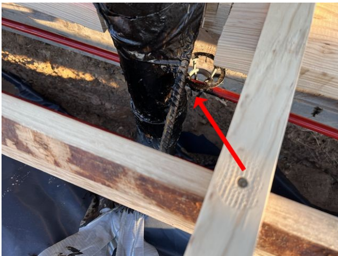
Cable clearance at the right drain pipe at garage
