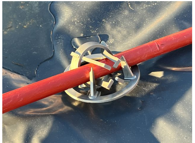
Damaged chair at garage interior pad
