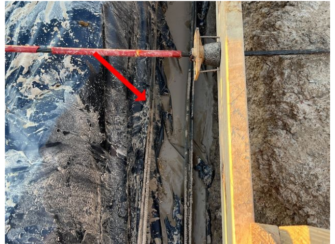
Rebar contact at rear patio pad at perimeter beam
