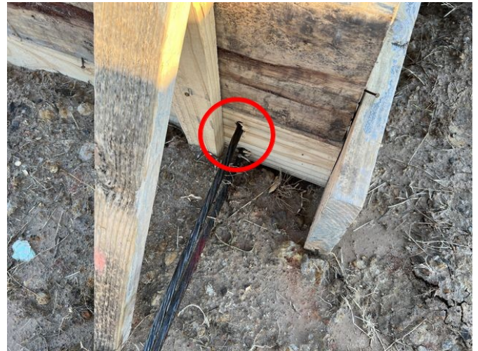
Cat heads missing at post tension cables at perimeter
