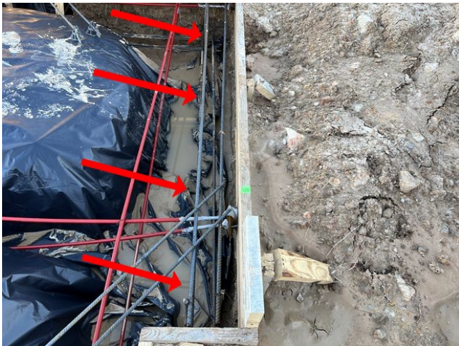
Stirrups missing at front porch rebar beams
