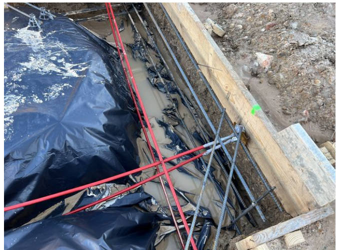
Excessive water standing at perimeter beams
