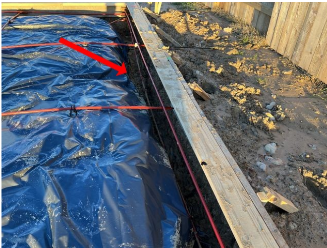
Cave-in/erosion at right perimeter beam
