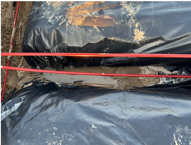
Standing water at footings
