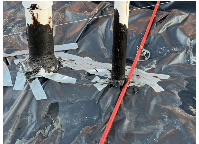
Cable contact drain pipe at interior pad rear garage
