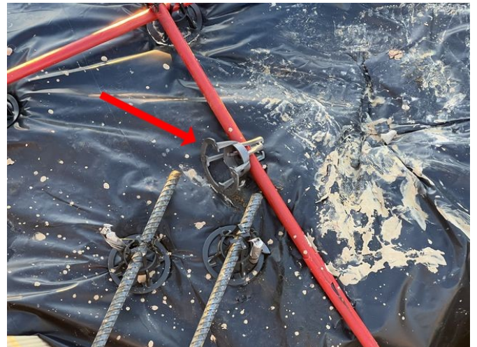
Damaged cable chair rear patio pad
