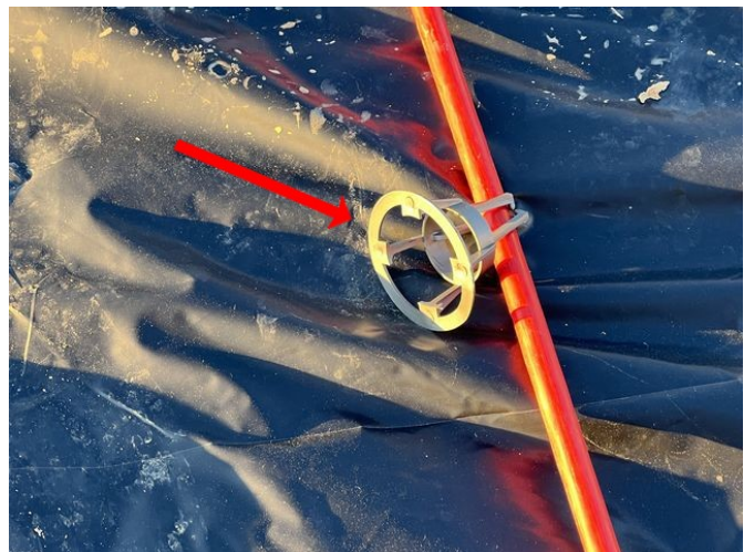
Several cable chairs shifted at the interior pads
