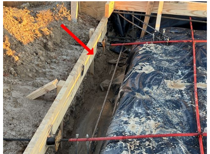
Cave-in/erosion at rear perimeter beam
