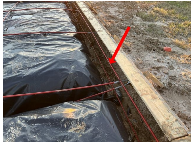
Cave-in/erosion at left perimeter beam
