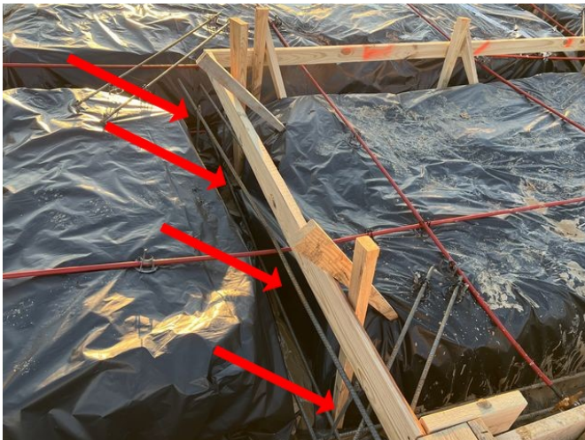
Stirrups missing rear patio rebar beam
