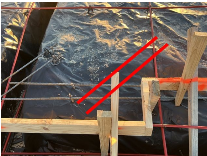
Re-entrant rebar missing interior corner rear patio
