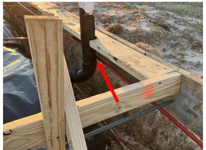
Cable contact drain left perimeter beam
