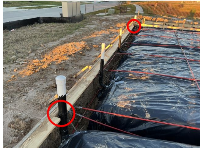
PVC drains encroach brick ledge left perimeter
