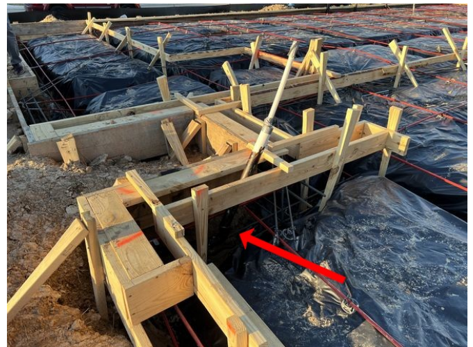
Waterline conduit detached left garage wall
