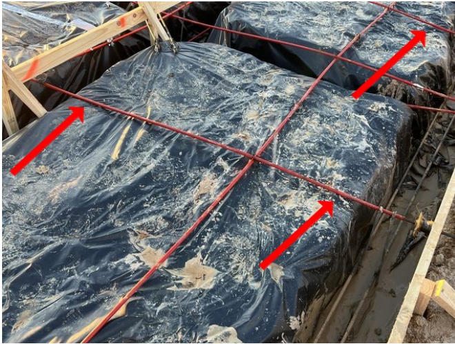
Cable chairs missing rear patio pads
