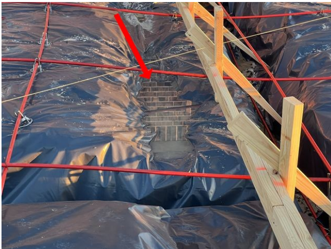
Standing water interior pads
