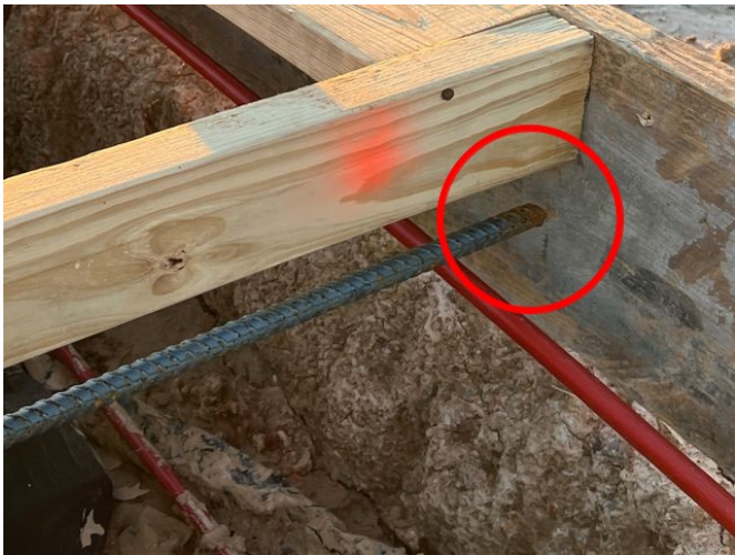
Rebar clearance left perimeter form at rear patio
