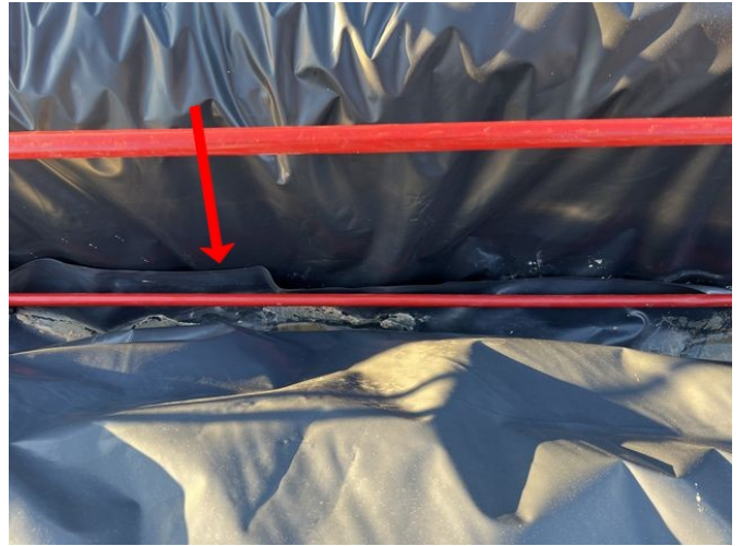
Poly overlap seam not taped at the interior beam
