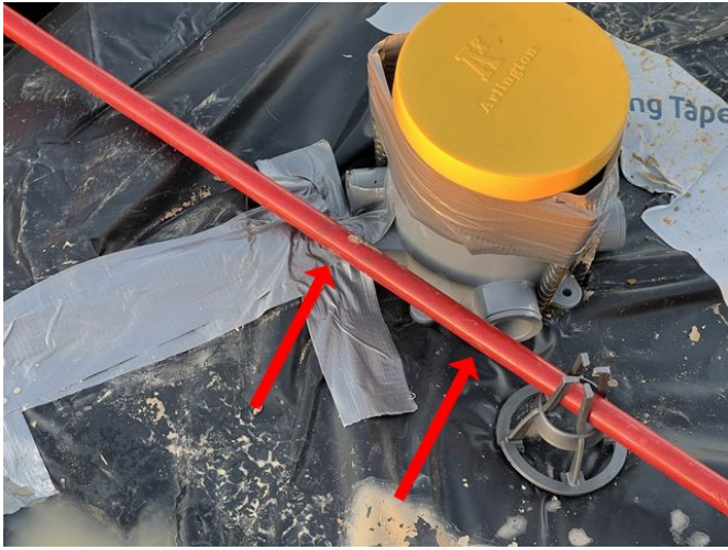
Cable contact floor plug housing and conduit
