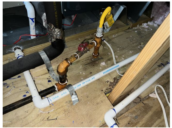
Gas pipe rusted left furnace in attic
