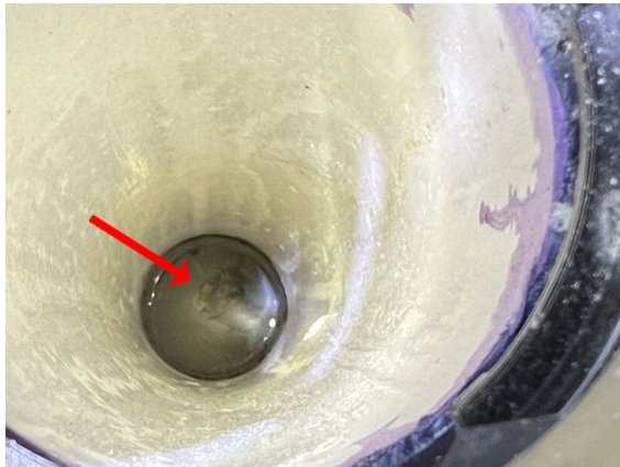
Debris master shower drain line
