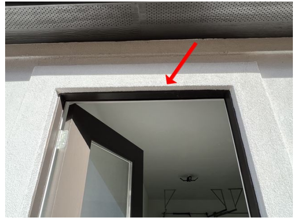
Z-flashing missing above left garage door
