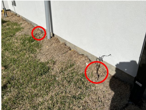
Ground rods not driven below grade
