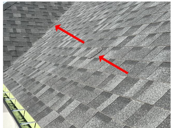
Construction debris left roof slope
