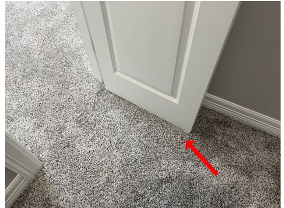
Door drags floor rear guest bed closet
