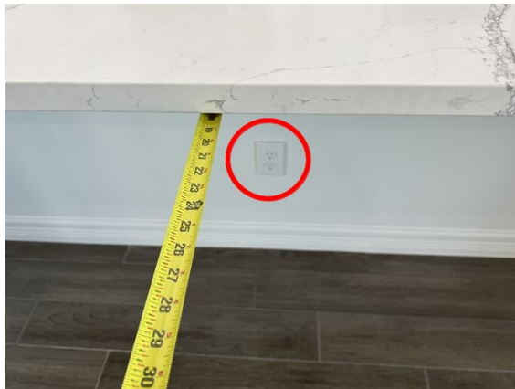
Receptacle under island overhang > 6"
