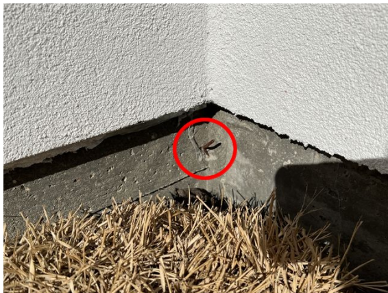
Exposed buckle nail front guest bed at corner
