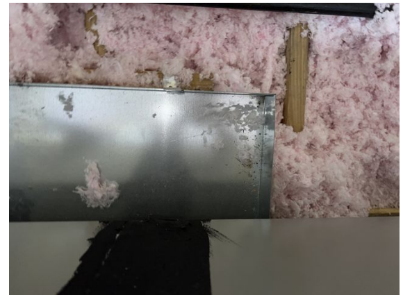
Debris right A/C drain pan
