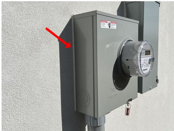
Required air space caulked at meter cabinet
