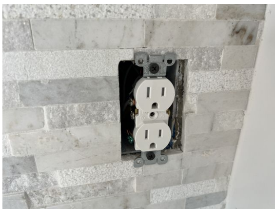
Spark rings missing kitchen backsplash outlets
