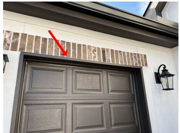
Z-flashing missing above garage door
