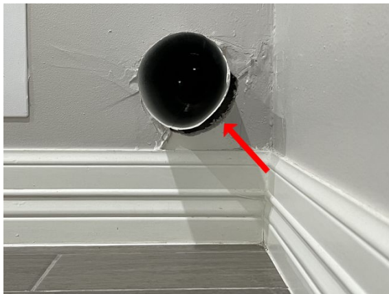
Hole drywall at dryer vent pipe
