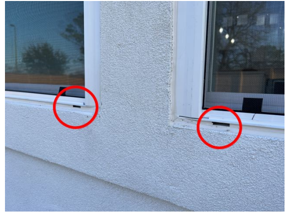
Drain port covers missing at several windows
