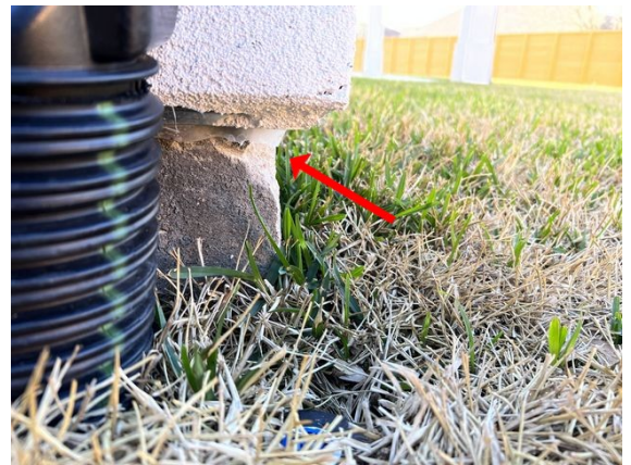
Corner missing right rear master bedroom slab
