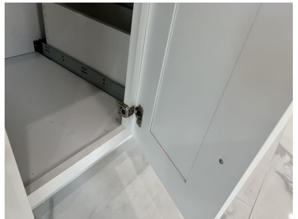
Master bathroom cabinet door binding
