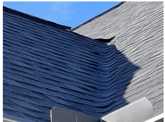
Cupping shingles front roof slope
