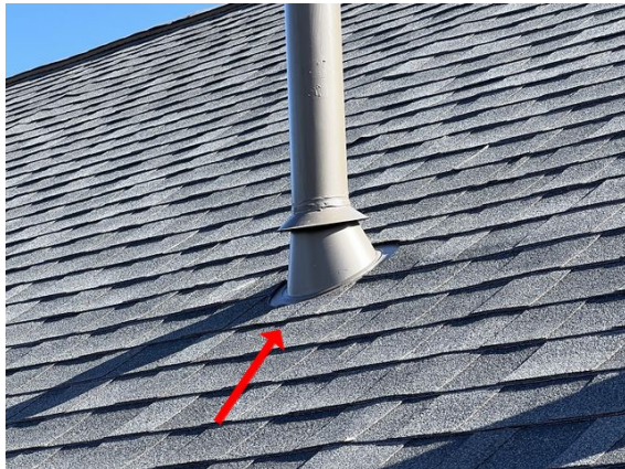
Improper shingle installation furnace roof jack
