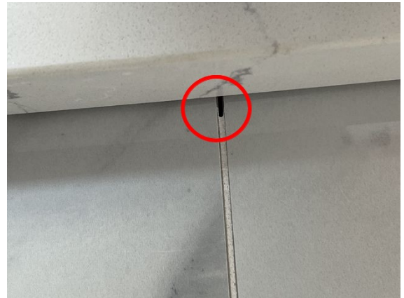
Tile grout missing under master shower seat
