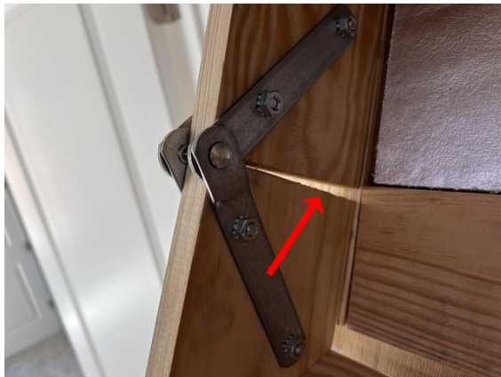
Attic ladder not properly trimmed
