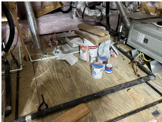
Attic deck not clear of obstructions
