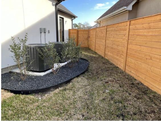
Evidence of ponding water left dwelling
