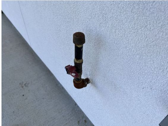
Gas pipe rusted rear patio
