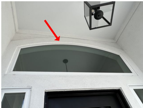
Z-flashing missing above entry arched window
