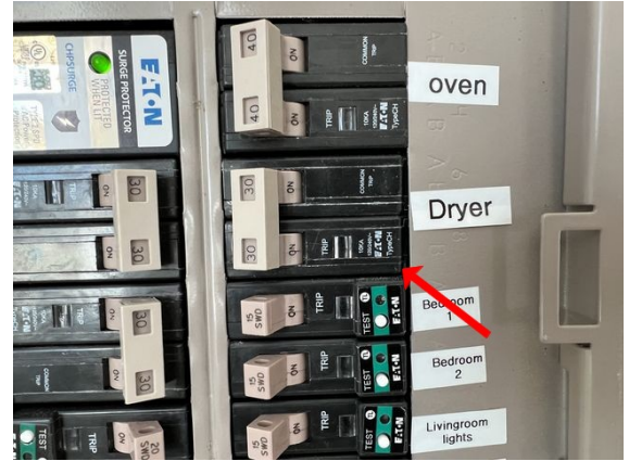
Dryer circuit breaker not GFCI protected
