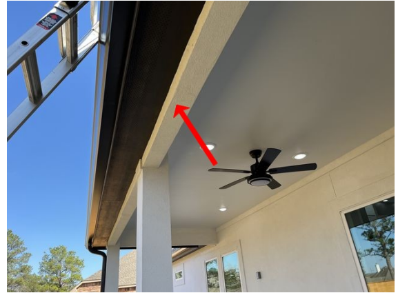
No drainage plane at rear patio beams
