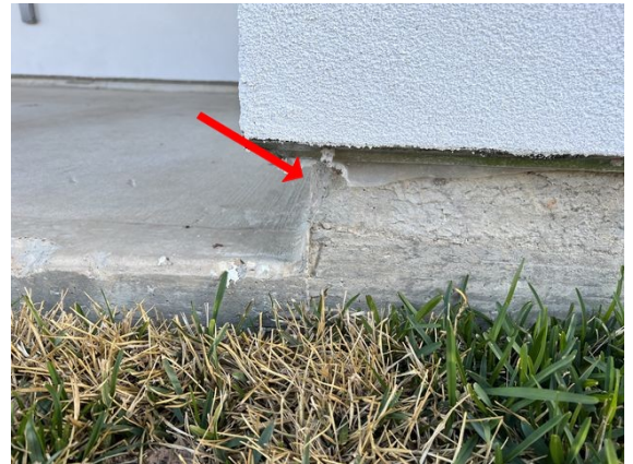
Corner missing right rear breakfast room slab
