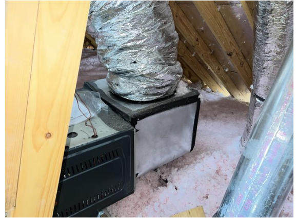
No fresh air intake at A/C return
