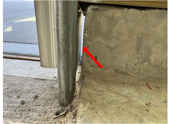
Gaps garage door jamb and slab stem walls
