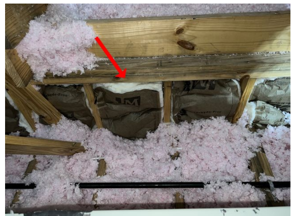
Insulation batts installed improperly attic walls
