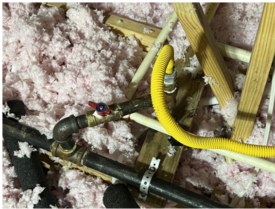
Gas odor at the water heater in the attic
