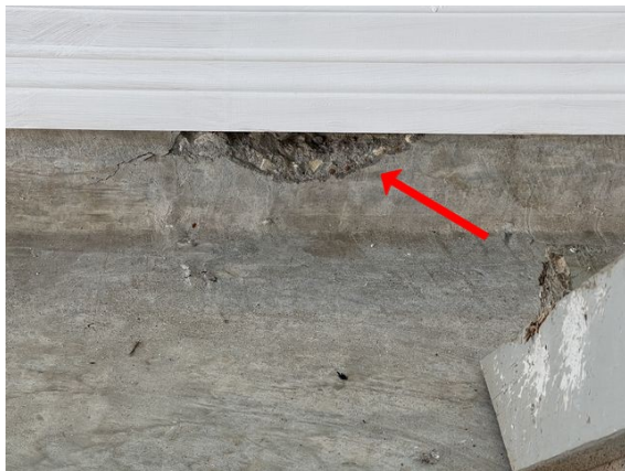
Concrete spall front garage stem wall
