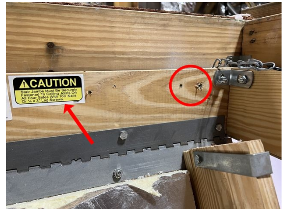
Improper fasteners at attic ladder frame
