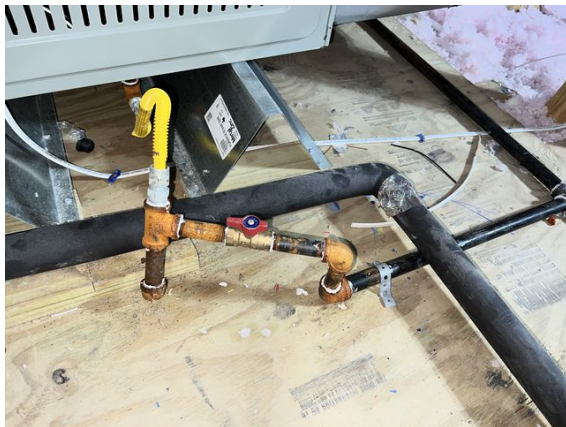
gap pipe rusted right water heater in attic
