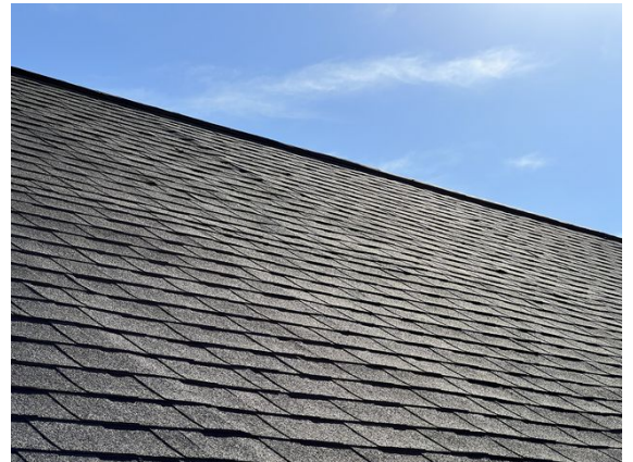
Cupping shingles rear roof slope
