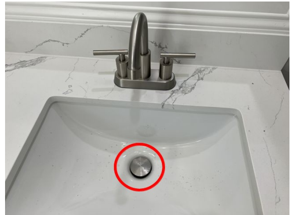
Sink stopper not working front guest bathroom
