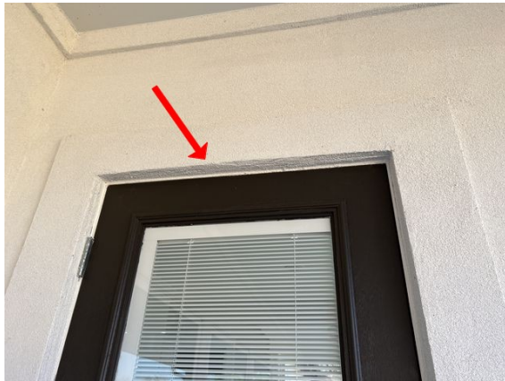
Z-flashing missing above rear patio door
