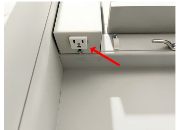
Ironing board receptacle not GFCI
