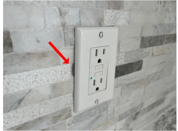
Backsplash tile missing at GFCI receptacle
