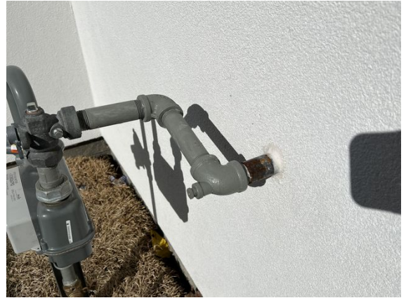
Gas pipe rusted at meter
