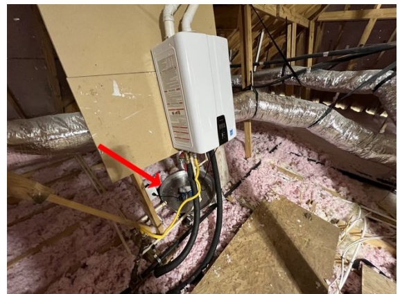
Water heater pan not position under the unit
