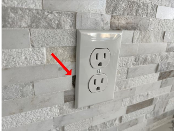
Backsplash tile missing at receptacle
