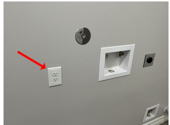
Washing machine receptacle not GFCI
