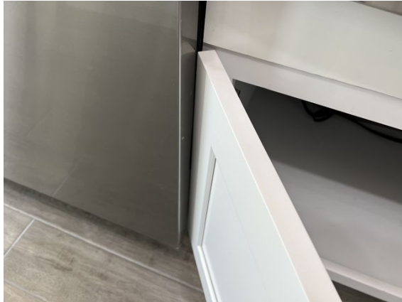
Kitchen cabinet door binding at dishwasher
