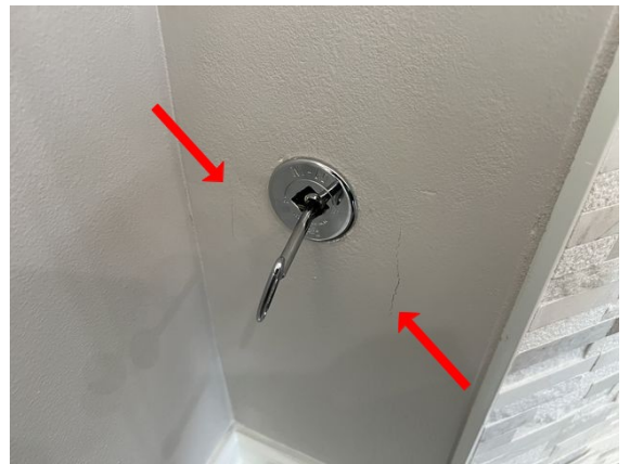
Drywall cracks at fireplace gas valve
