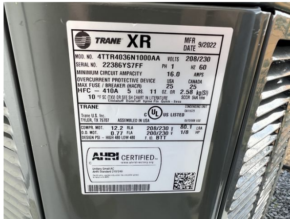
A/C condensing unit labeling
