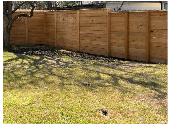
Evidence of ponding water rear yard
