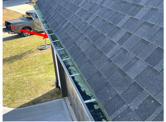
Standing water right garage gutter
