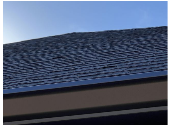
Cupping shingles right roof slope
