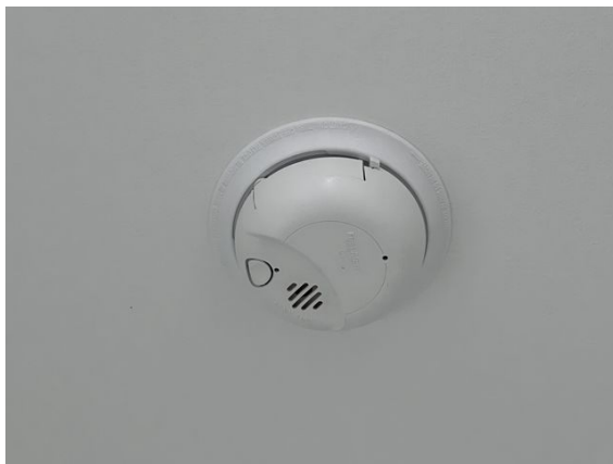
Smoke alarm not CO exterior rear bed
