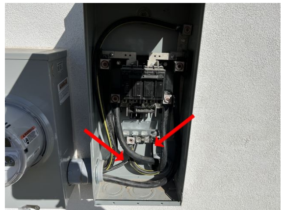
Black sheathed grounds not marked green
