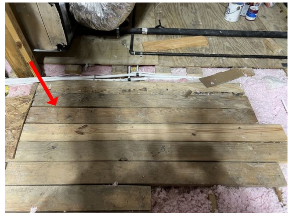
Loose attic decking at several locations
