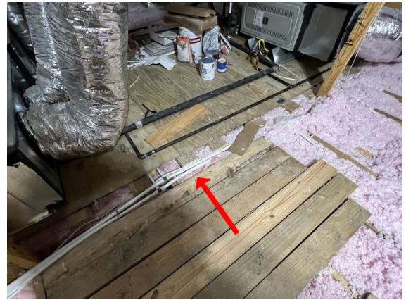
Gaps attic deck at furnaces
