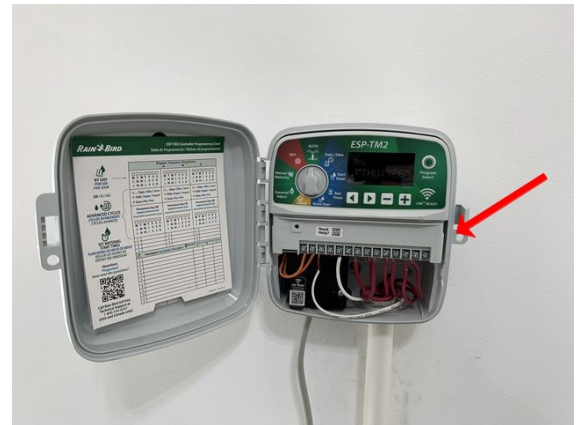
Sprinkler interior cover panel missing
