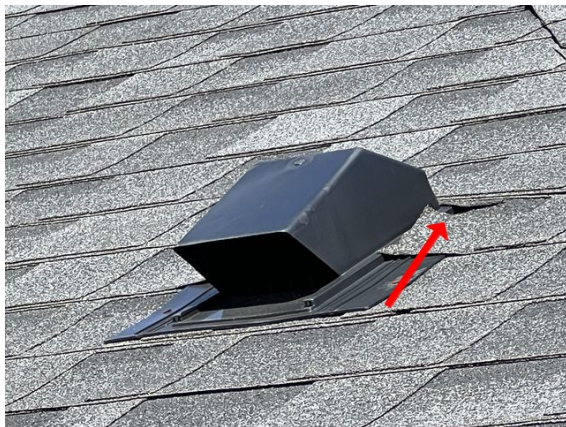
Damaged shingle tab left slope roof jack
