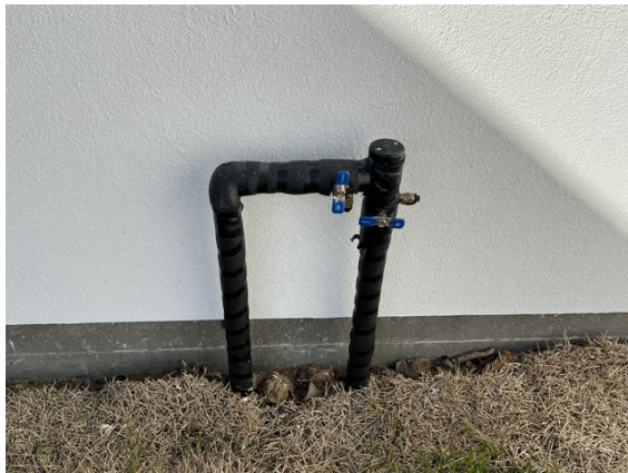
Sprinkler system winterized, not operated
