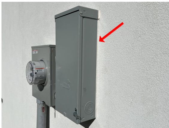
Required air space caulked at panelboard
