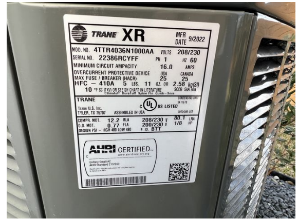
A/C condensing unit labeling
