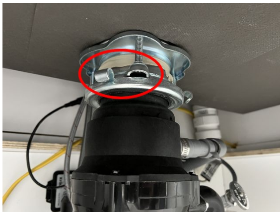
Disposal clamp not locked into place
