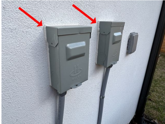
Required air space caulked at A/C disconnects
