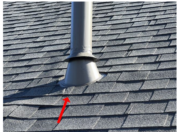
Improper shingle installation furnace roof jack
