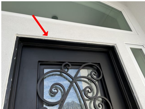
No z-flashing above front entry door
