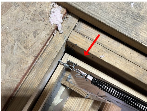
Attic ladder not poly sealed at ceiling joists
