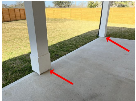
Stucco clearance base rear patio columns
