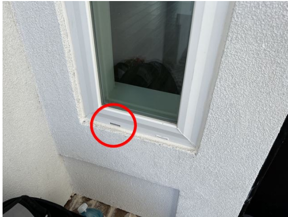
Drain port covers missing at several windows
