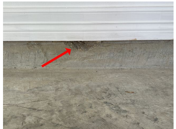
Concrete spall slab rear garage wall
