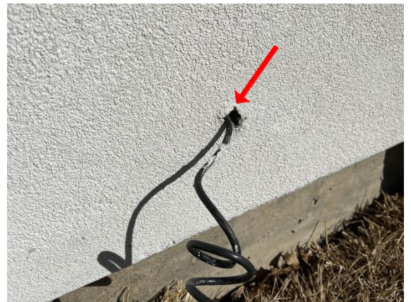
Seal penetration grounding conductor
