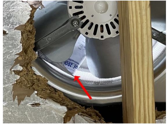
Debris in the attic mechanical fan
