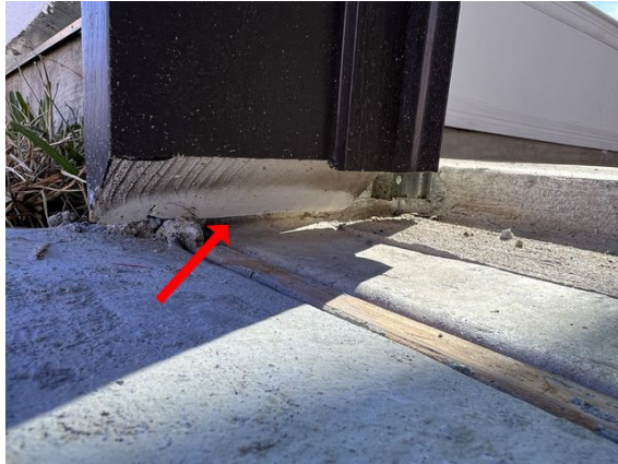
Garage door jamb end cuts not properly painted
