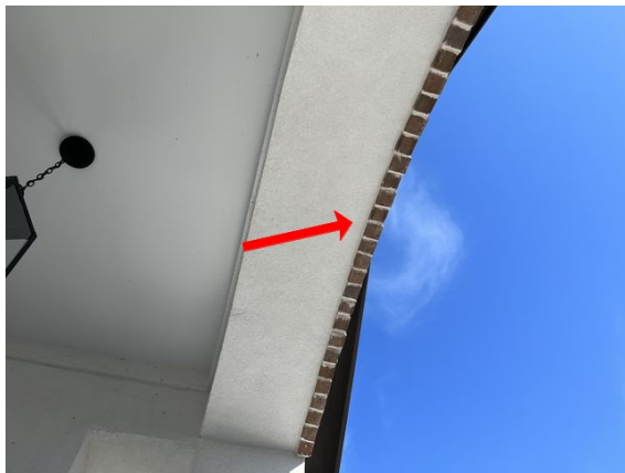
No drainage plane front porch arch
