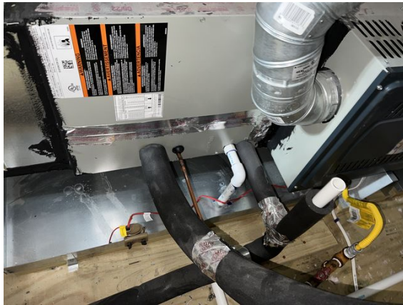
Penetrations not sealed left evaporator
