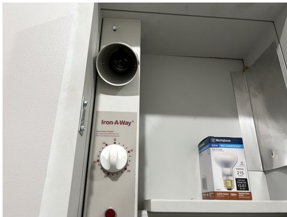
Light missing ironing board fixture
