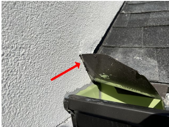
Kickout flashing not caulked at stucco
