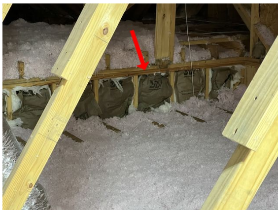
Insulation batts installed improperly attic walls
