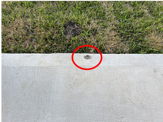
Honeycomb rear patio slab
