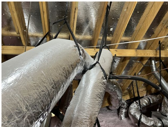
Separate ductwork where touching at attic
