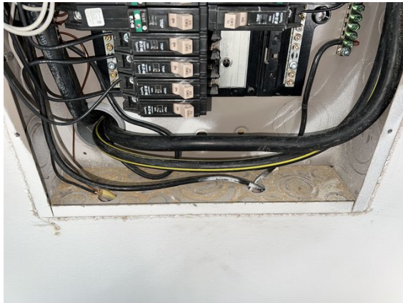
Debris bottom panelboard
