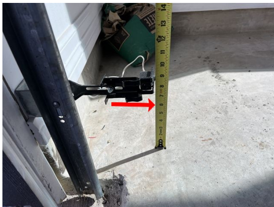
Garage sensors too high above floor
