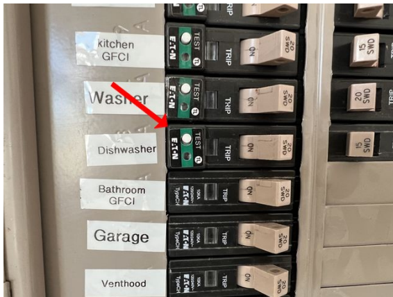
Dishwasher circuit breaker
