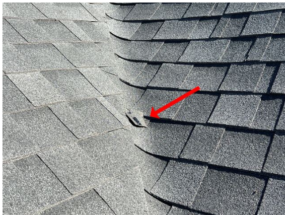
Construction debris left roof slope
