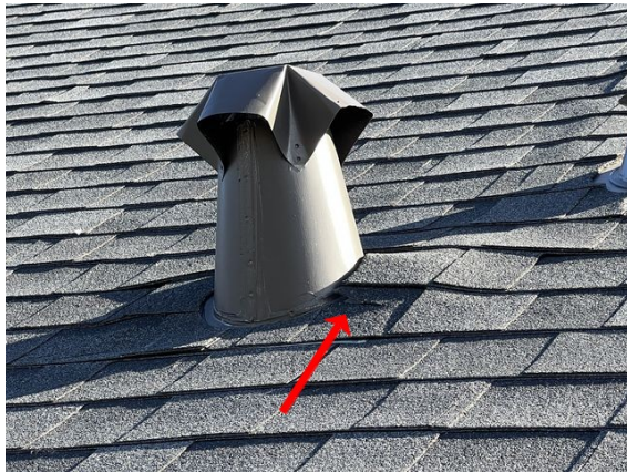
Raised shingle surface, cracked tap range hood
