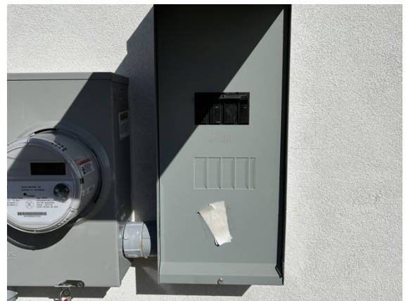
Label missing dead front cover
