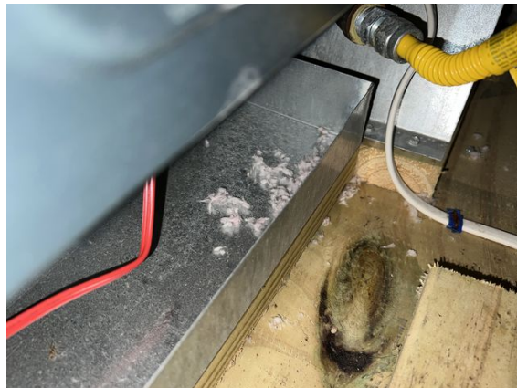
Debris left A/C drain pan
