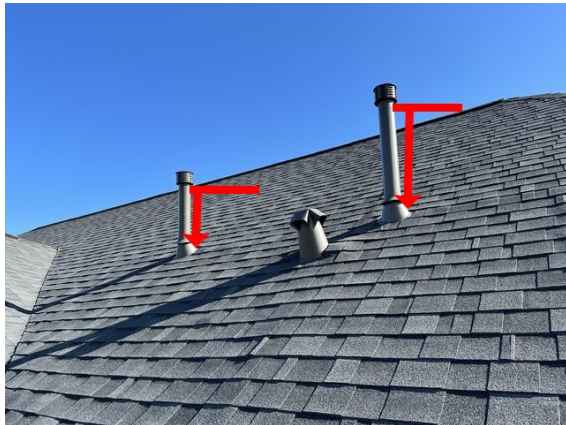
Furnace vent pipes too short for roof slope
