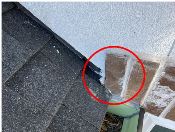
Kickout flashing missing garage roof at wall
