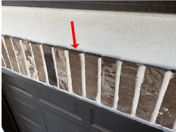
Brick not sealed above garage door
