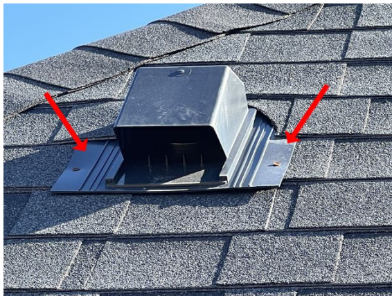
Shingles not installed over sides rear roof jack
