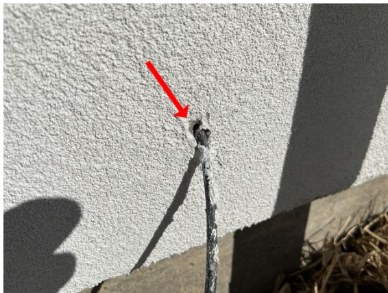
Seal penetration grounding conductor
